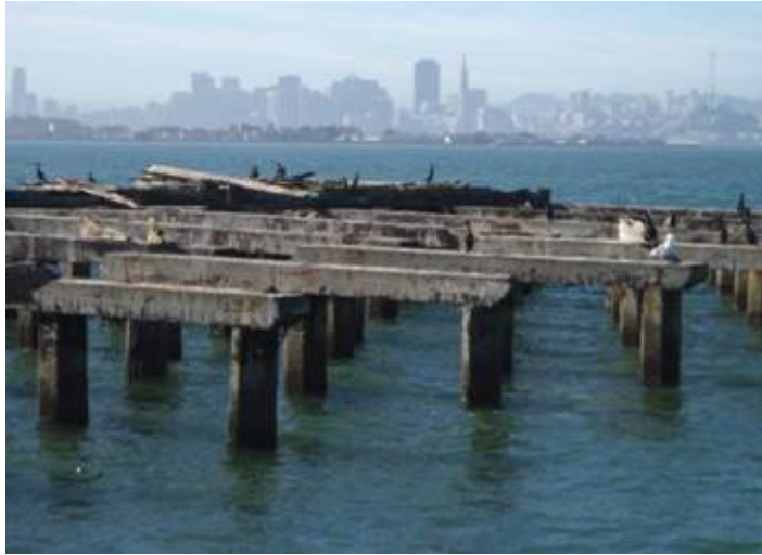
Figure 7: Tip of the derelict portion of the Berkeley Pier. Photo by Steve Hampton, CDFG.
