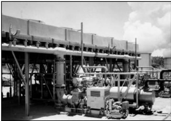
Figure 13. Tarawera 1.25-MWe binary unit at Kawerau, New Zealand.
