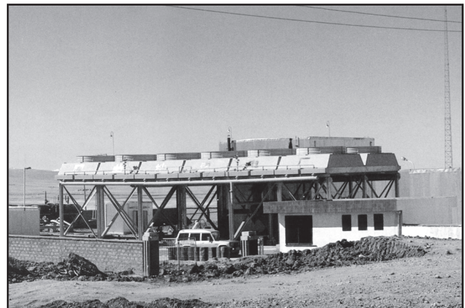
Figure 11. Nagqu 1.0-MWe power plant in Tibet at 14,850 ft. (4,526 m) elevation.
