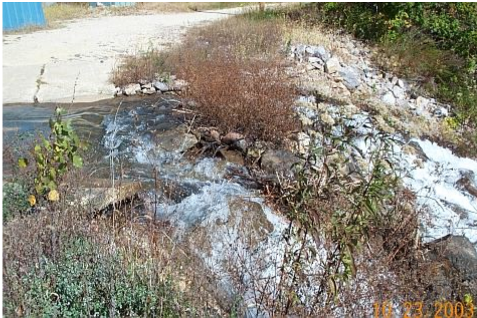
Figure 3.8 - Overflow of the seepage collection Pond before liner installation (2003 FERC Operation Inspection Report)
