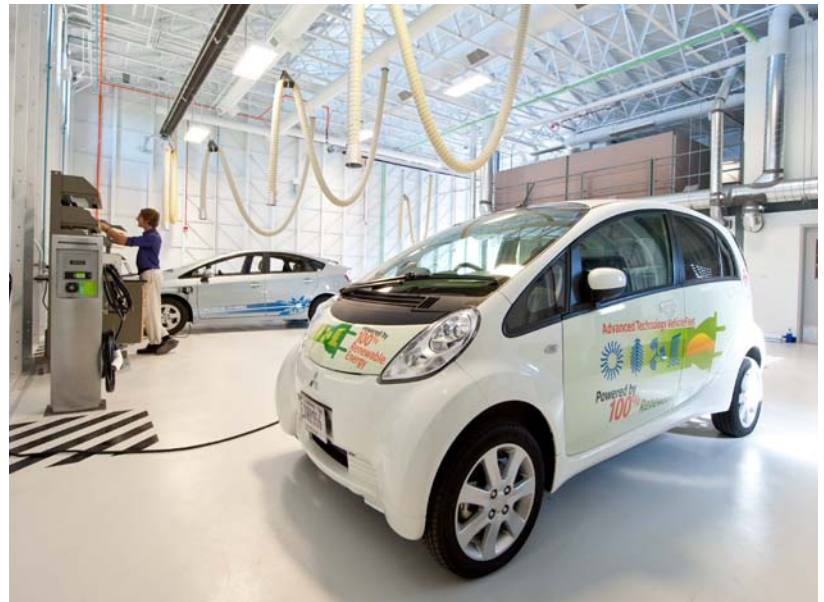
PEV charging in the VTIF. Photo by Dennis Schroeder, NREL/PIX 19758
