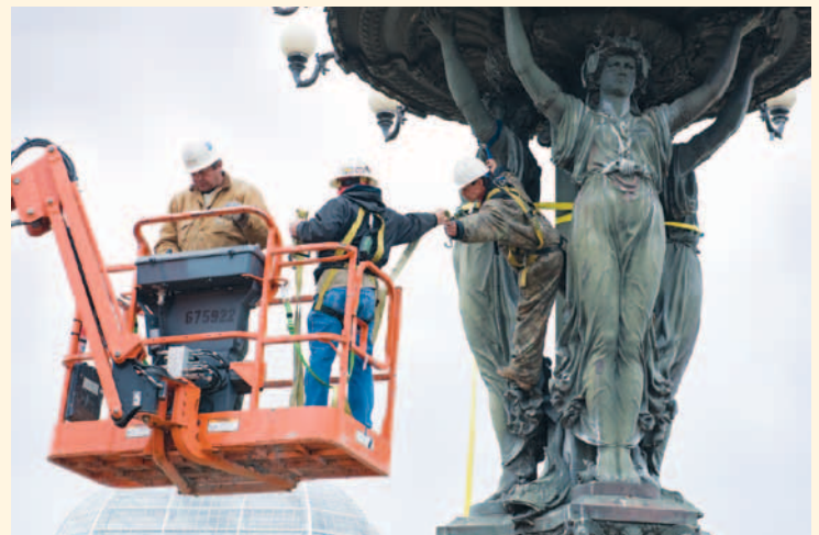
The historic 1876 Bartholdi Fountain was disassembled, removed by crane, and sent to an architectural metal specialist to restore the sculpture to its original beauty and update it with energy efficient technology.
