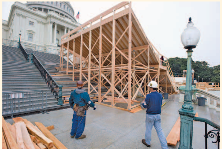
The AOC is responsible for building the Inaugural platform where the President of the United States is sworn in. The platform is made entirely of lumber to protect the surfaces of the Capitol.
