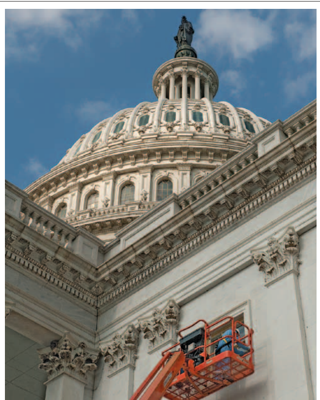
The AOC maintained the Capitol by preparing, priming, and repainting the exterior stone surfaces and windows during the Fiscal Year to prevent moisture penetration and corrosion.
