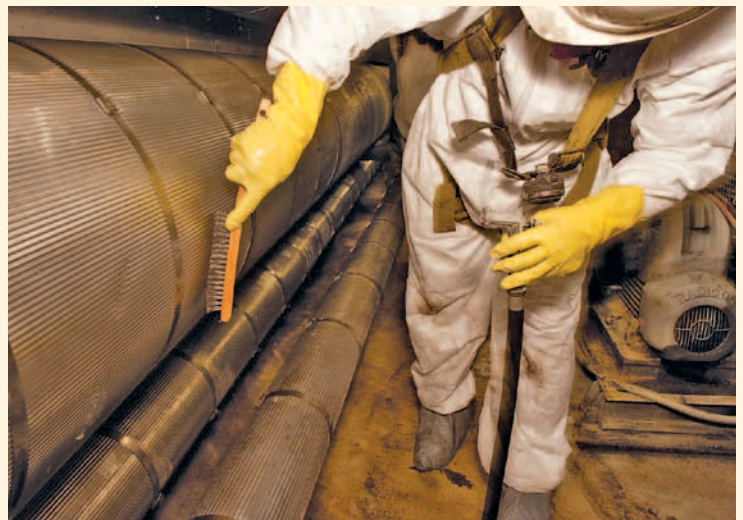
The AOC made strides in abating utility tunnel health and safety issues during the Fiscal Year and currently estimates the tunnel abatement work will cost slightly over $176 million.
