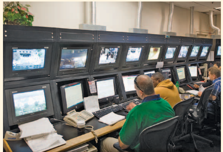
The AOC has begun work on the design and construction of a primary and mirror site data center to support the U.S. Capitol Police's program to modernize their radio system.
