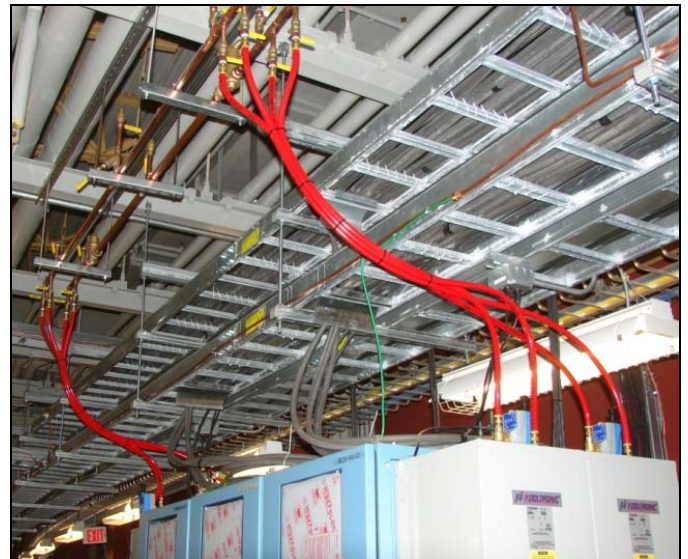
Figure 1. Racks with process chilled water (PCW) connections.
