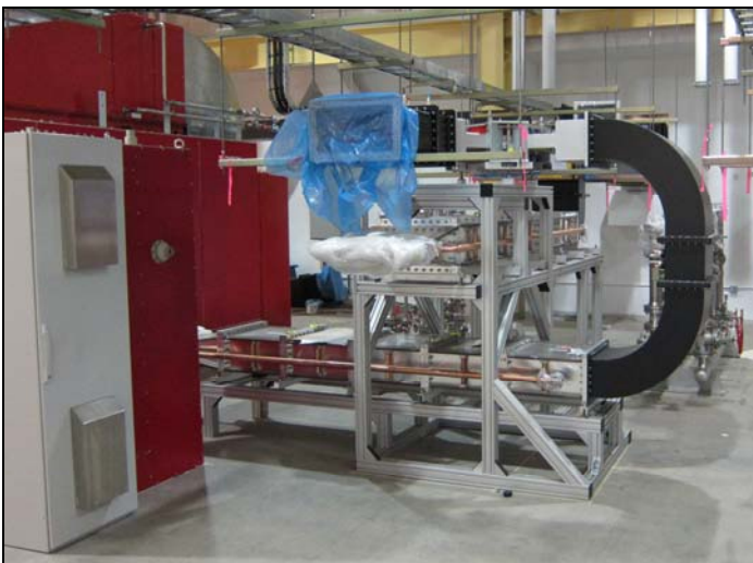
Figure 7. Klystron HVPS, control rack, and circulator/load waveguide network.
