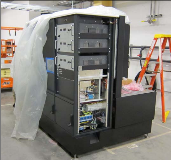
Figure 6. Solid state modulator in the NSLS-II klystron gallery.
