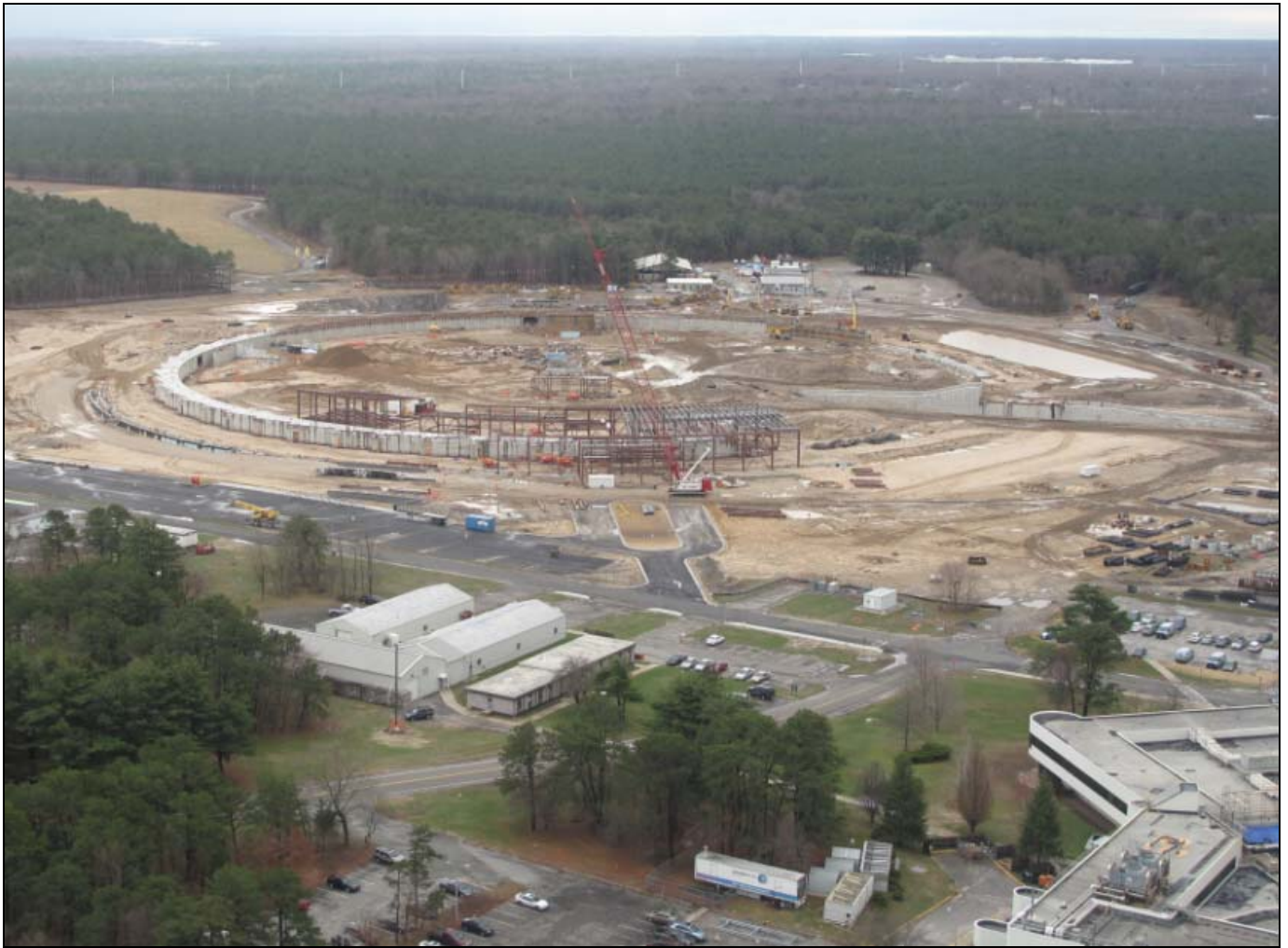
Erection of structural steel for pentant 1 progresses rapidly as the form and scale of the Ring Building take shape.
