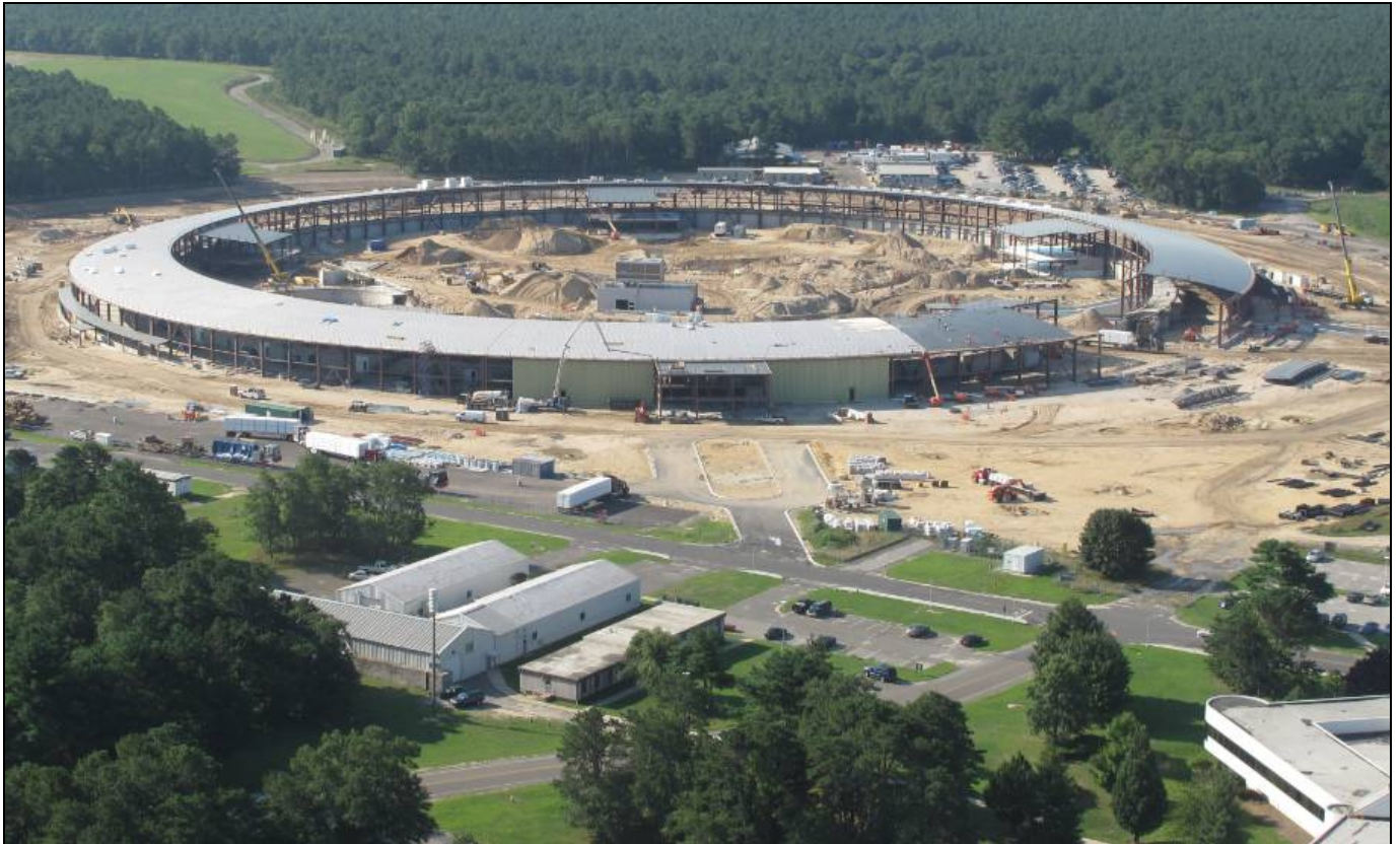
July 30: Roof surfacing continues, and insulated panels (minus their outer sheathing) begin to appear on the walls of pentant 1.
