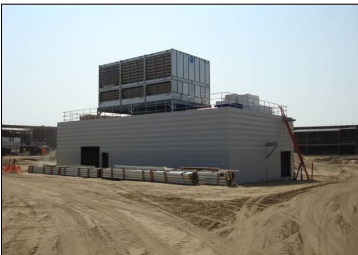
Figure 7. Cooling tower and process water building.
