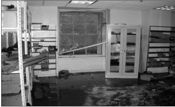
Destroyed equipment in the basement of the IRS Headquarters Building after flooding
