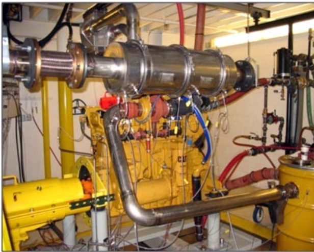
FIGURE 1. Caterpillar C9 Retrofitted With Emission Control System
