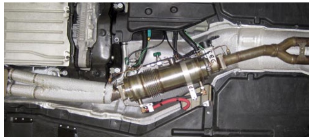
FIGURE 2. BMW X6 TEG Installation, Courtesy of the BMW Group
