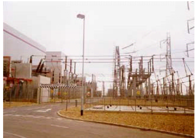
Figure 2. Goal is to accelerate application in the field such as at the substation shown.
