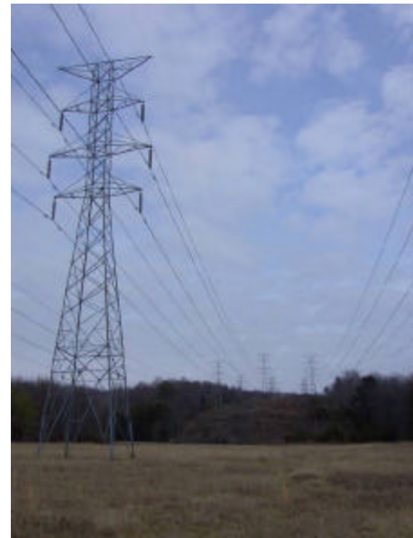
Figure 1. A unique arrangement of transmission facilities at PCOT provides at-voltage and at-current transmission conductor testing flexibility.
