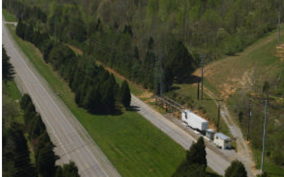
Figure 1. Aerial view of PCAT including its power supply and instrumentation trailers, transmission line structures and current conductor under test.
