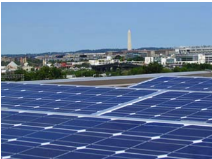
Photo courtesy of SolarCity. Solar panels on roof of DCHA's Sheridan Station.
