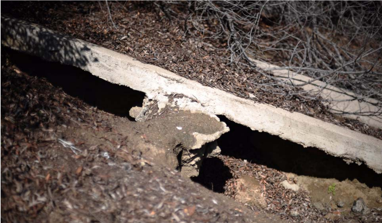
Photo 3-13. Undercutting of concrete chute.
