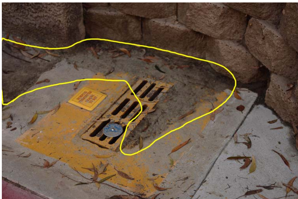
Photo 3-10. Drain showing sandy soil transported from hillside.
