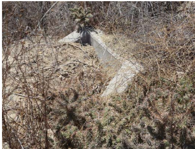
Photo 4-2. The City property to the north drains into Naval Medical Center San Diego property in several places. Some of these structures, like the one pictured above, is not well maintained and could result in future erosion problems.
