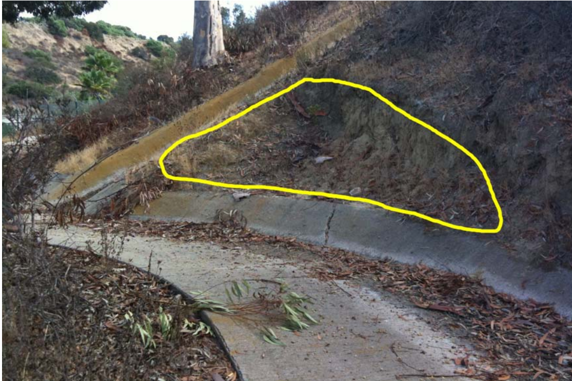
Photo 3-26. Erosion above and to the right of brow ditches on the eastern slope looking south.
