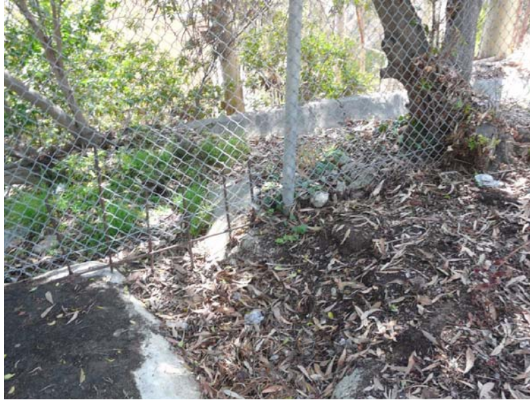
Photo 3-24. View from the City's side of the fence, where debris is entering NMCS D property and clogging the confluence of the two brook ditches. Note Brazilian pepper tree in upper left corner also blocking flow.
