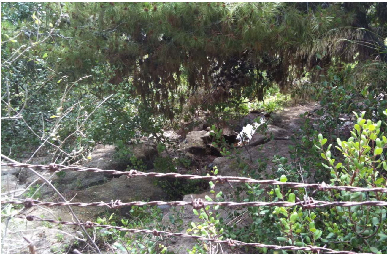
Photo 3-14. Minor erosion on city of San Diego property outside of fence.
