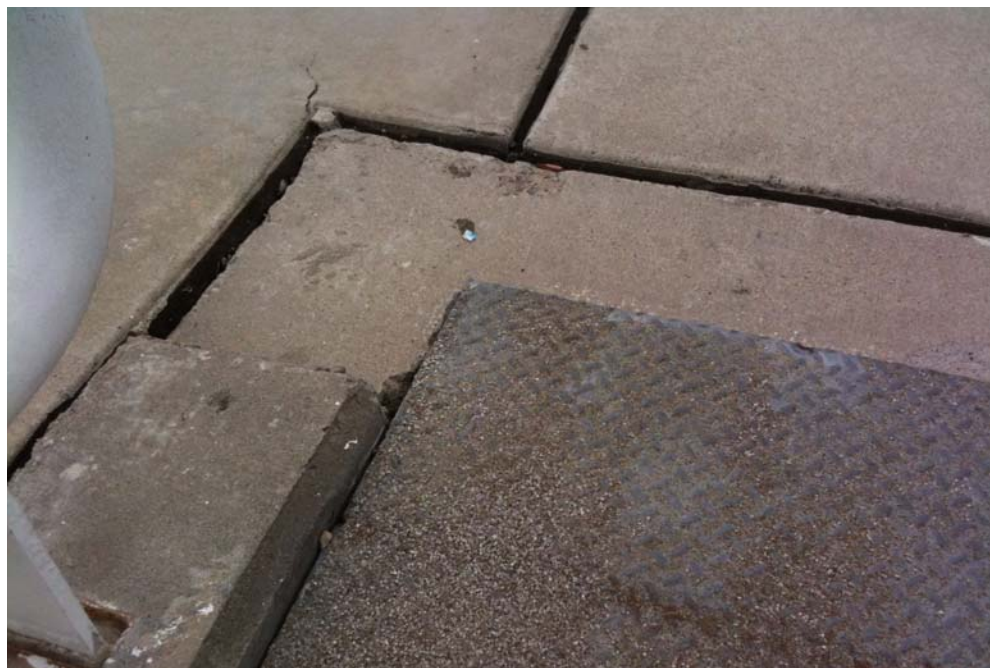
Photo 3-3. Concrete along walkway settling down over eroded area beneath.
