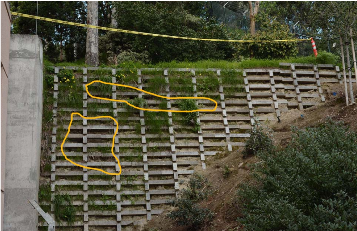
Photo 3-21. Areas (encircled) where crib wall is eroding from within.
