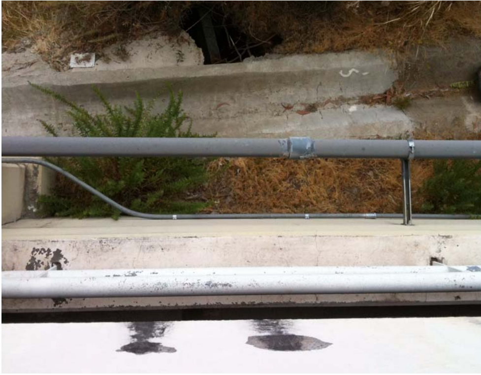
Photo 3-20. View looking down from the roof of the parking lot. Note drainage holes at bottom center and the eroded hole at top center.
