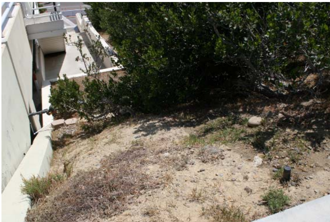
Figure 19. Bare area on Site 10.
