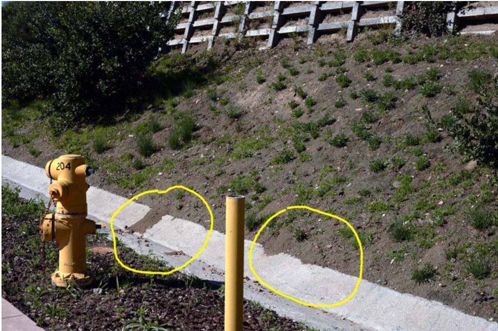
Photo 3-1. Slope lacking shrub cover beneath concrete bracing. Circled area shows soil movement.
