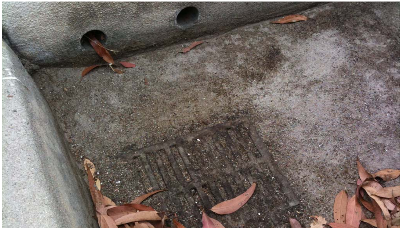
Photo 3-19. Note clogged drain, and ad hoc drainage holes at top.
