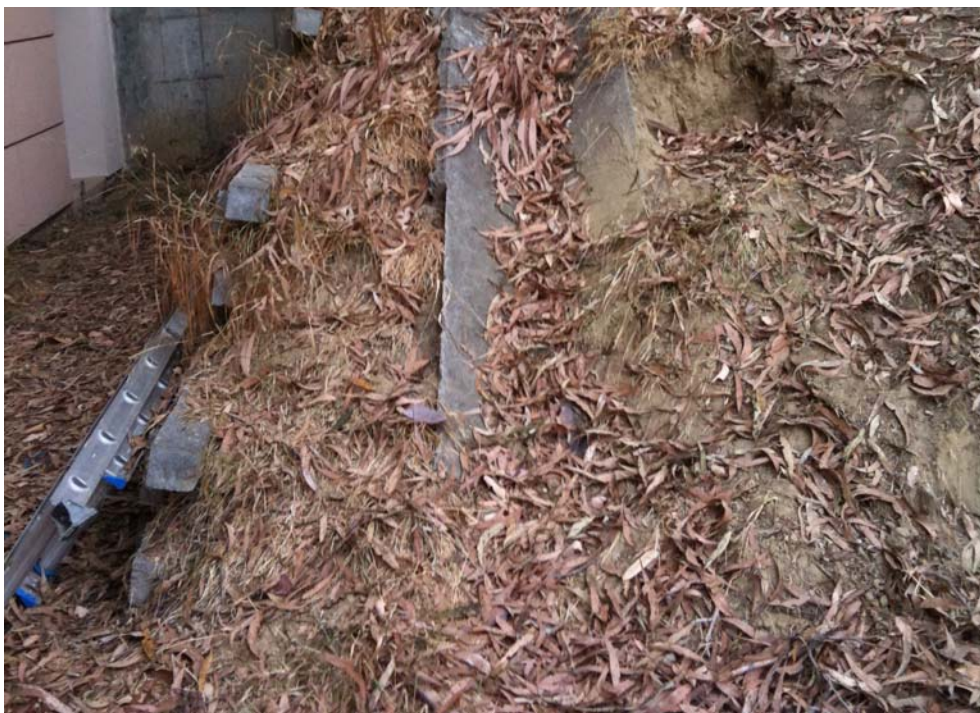
Photo 3-22. Source of erosion: a brow ditch is filled with debris.
