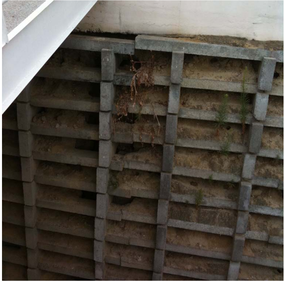
Photo 3-2. Photo showing erosion within crib-wall.
