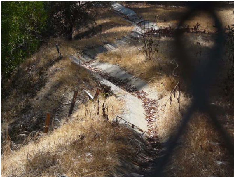
Photo 3-23. Brow ditch with soil eroding downslope.
