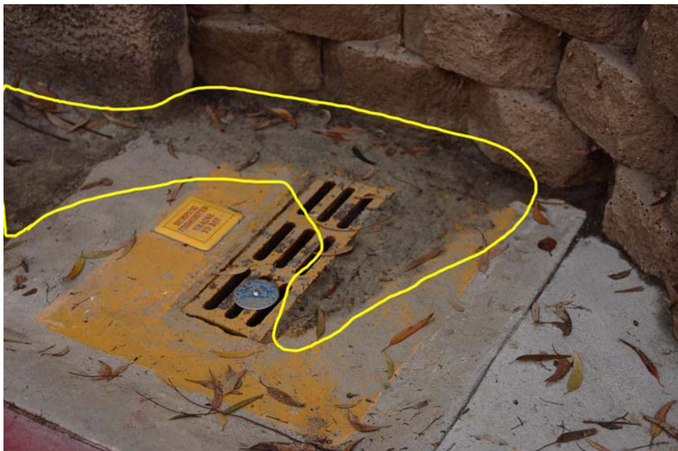
Photo 3-10. Drain showing sandy soil transported from hillside.
