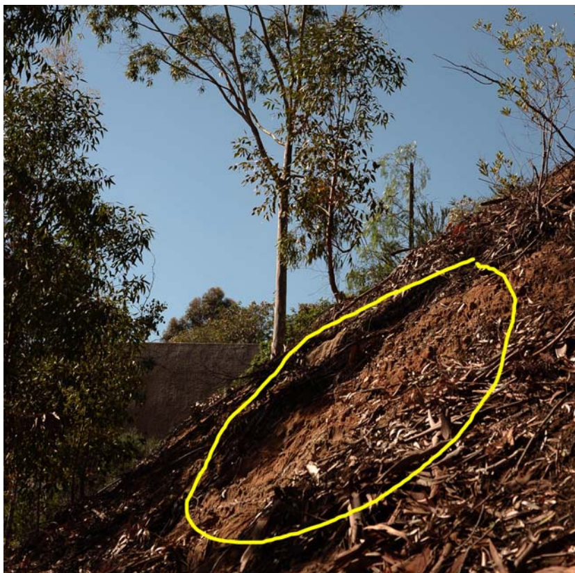
Photo 3-7. Exposed slope (encircled) outside the cover of eucalyptus trees.
