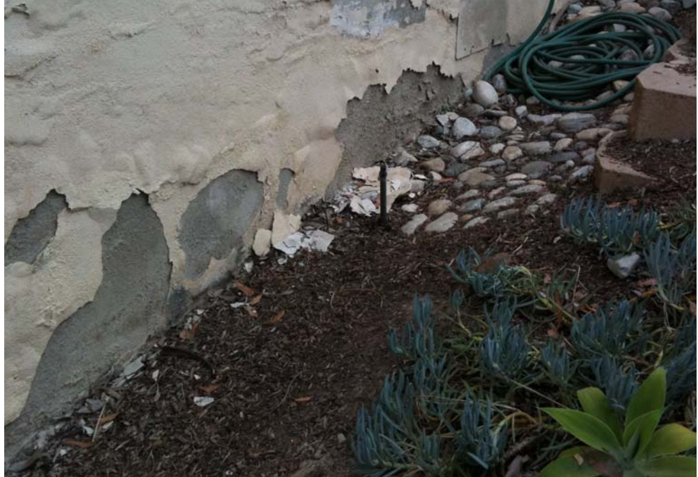
Photo 4-1. Ineffective sprinkler on the north side of the Fischer House directed to the wall (note premature wear on stucco) surrounded by drought tolerant ice plant.
