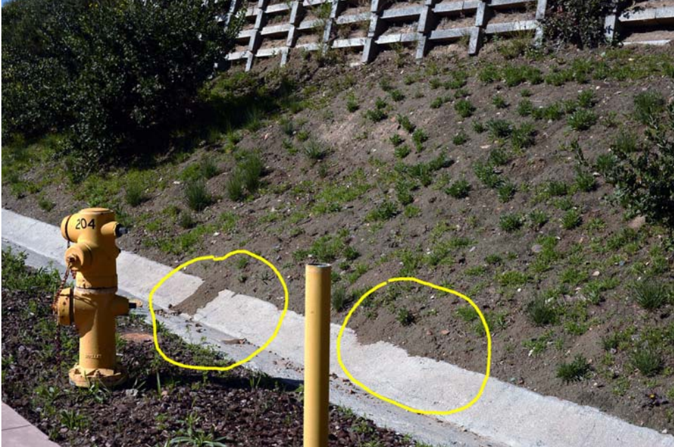
Photo 3-1. Slope lacking shrub cover beneath concrete bracing. Circled area shows soil movement.
