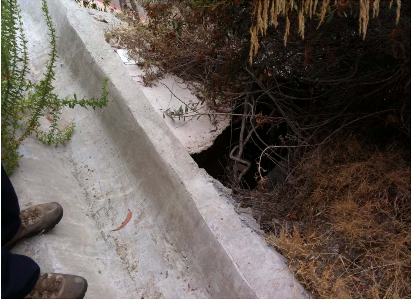
Photo 3-17. Point of entry of water, just outside the concrete drainage ditch.
