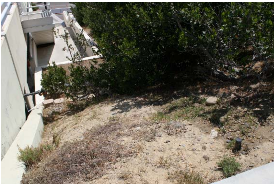
Figure 19. Bare area on Site 10.
