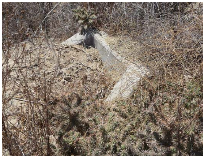
Photo 4-2. The City property to the north drains into Naval Medical Center San Diego property in several places. Some of these structures, like the one pictured above, is not well maintained and could result in future erosion problems.
