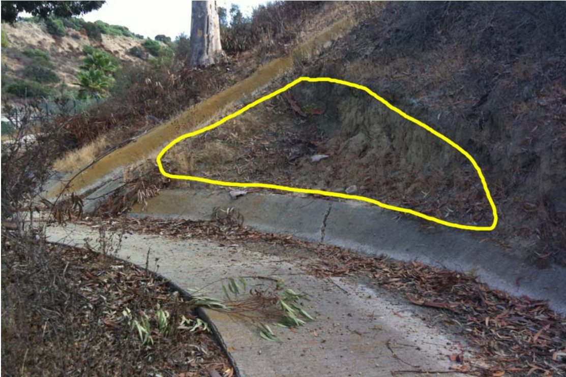
Photo 3-26. Erosion above and to the right of brow ditches on the eastern slope looking south.
