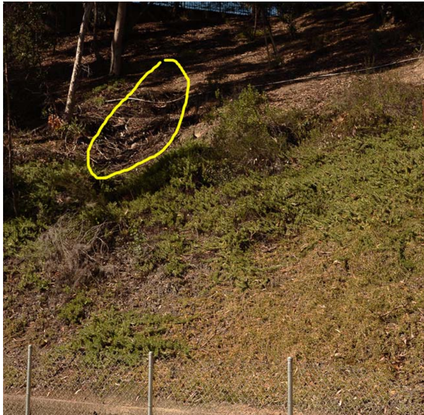
Photo 3-8. Large gully halfway upslope. Note broken PVC pipe (encircled) above and vegetation below.
