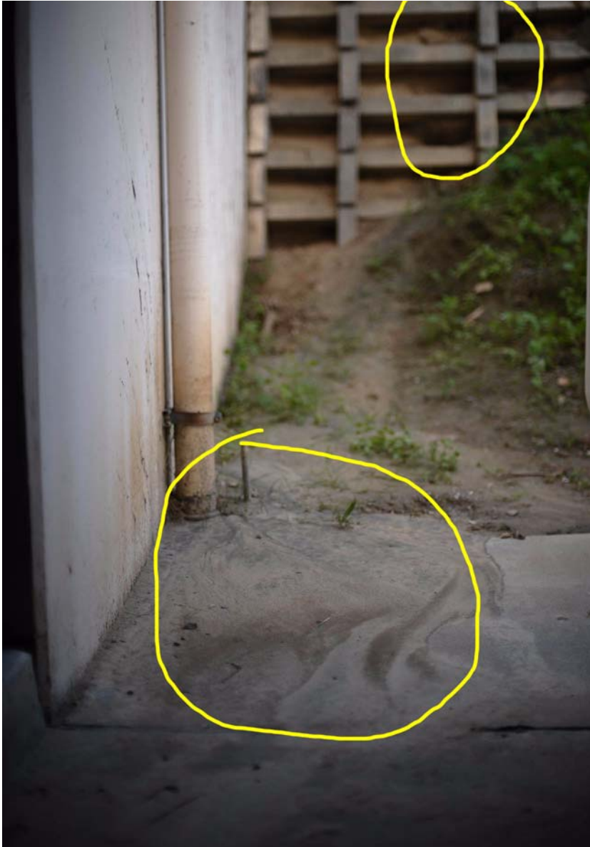
Photo 3-4. Smaller circle shows location of soil loss inside concrete bracing. Larger circle shows soil movement into the gutter system.
