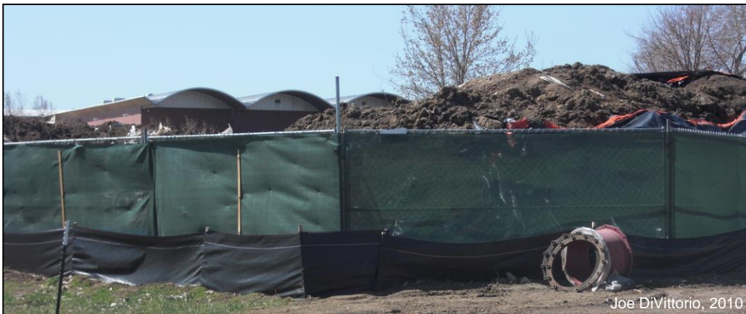
Figure A-4. Stockpiled fill material at a construction site enclosed by silt fencing to help control soil loss and the potential spread of foreign species. Black plastic covering (seen in upper right corner) has been pulled back to allow machine work (photo courtesy of Joe DiVittorio, 2010).
