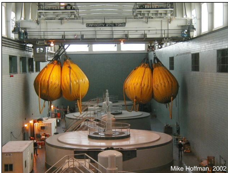
Figure 12. Crane being tested at a Tennessee Valley Authority powerplant using water weight bags™ (photo by Mike Hoffman; photo courtesy of Jim Jota, Imes, Inc., 2002).
