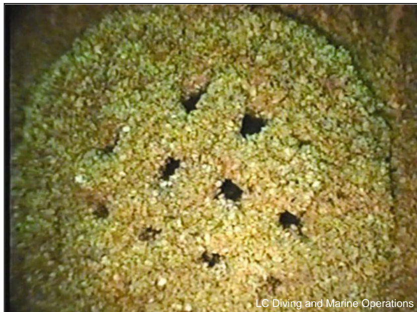
Figure 9. Underwater photo showing mussels covering the Davis Dam domestic water intake grate (photo courtesy of LC Diving and Marine Operations, 2008).
