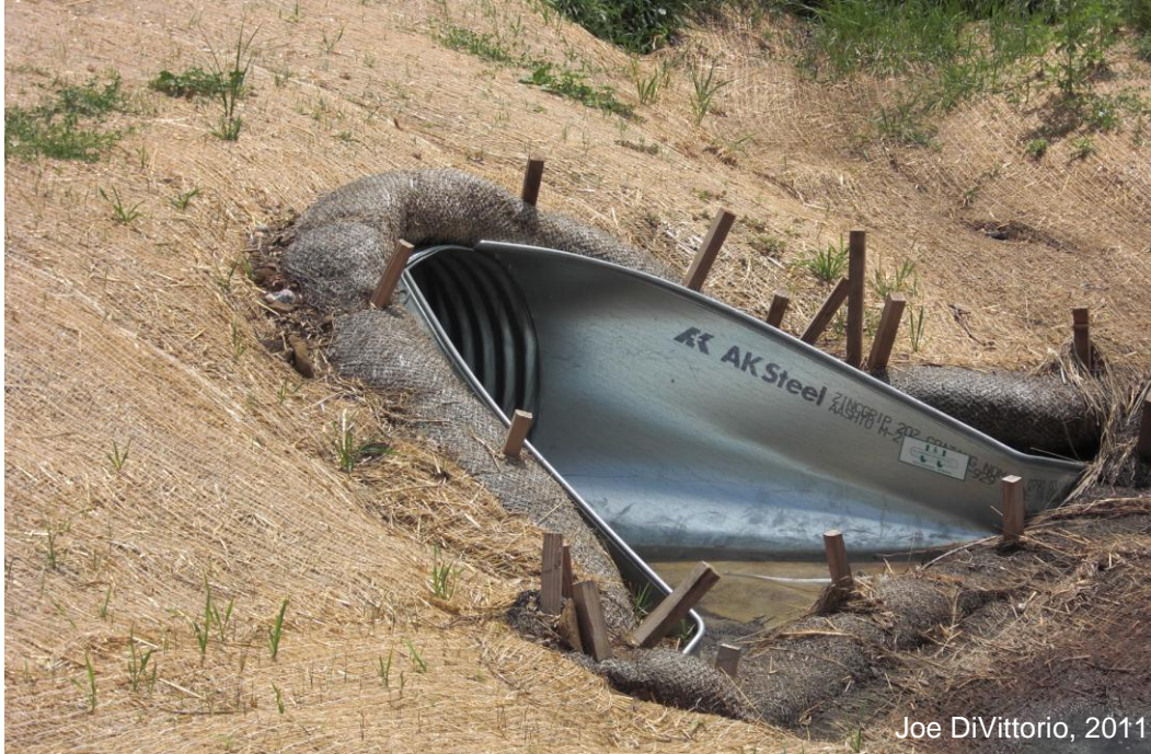
Figure A-1. Straw is used as a mulch and in sediment logs to control erosion. Here, sediment logs (or wattles) are shown staked around a culvert (photo courtesy of Joe DiVittorio, 2011).
