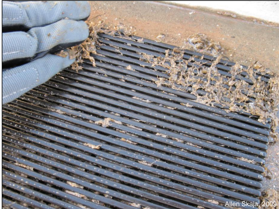
Figure B-14. This is an example of a foul release coating that has been in the water for 18 months. Mussels and algae growth may attach to the surface under certain flow rates; however, they are easily removed (photo courtesy of Allen Skaja, 2009).
