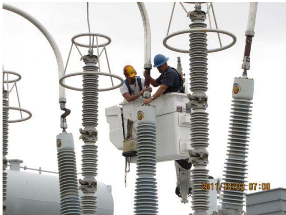
Electrical Utilities completes preventative maintenance on the A6 substation
