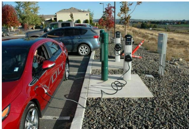
Electric Charging Station at Stevens Center
