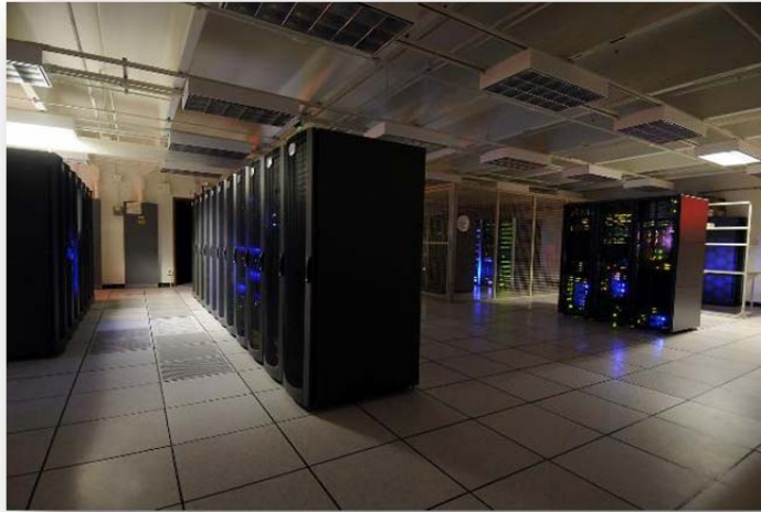
Data Center Photo
