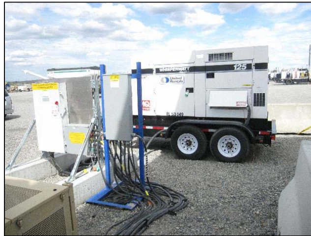
250 amp Main Service Disconnect and generator swap out
