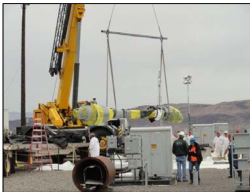
Failed 106 AN supernate pump being loaded for shipment to ERDF
