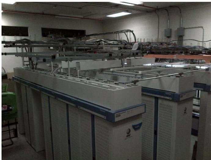
5ESS Units Being Replaced by the VoIP Upgrades
