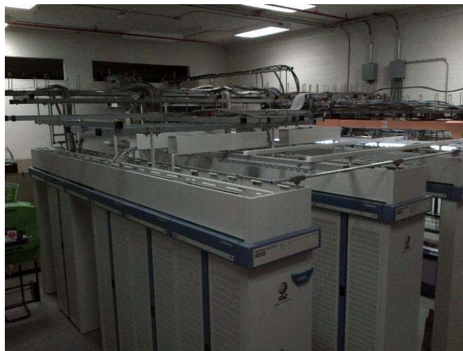
Transition of 5ESS Units to Voice Over Internet Protocol (VoIP) Continues
