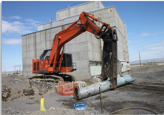
Demolition of piping and a water tunnel in the 100K Area continues
