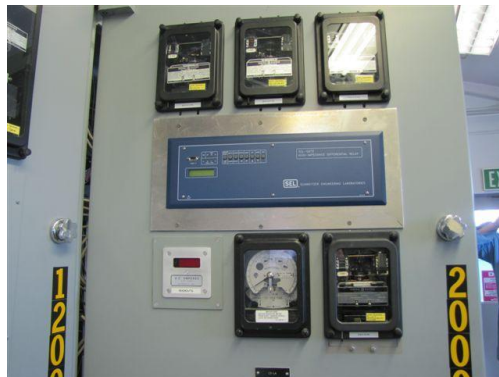
Electrical Utilities installed new Solid State Relay Devices.
