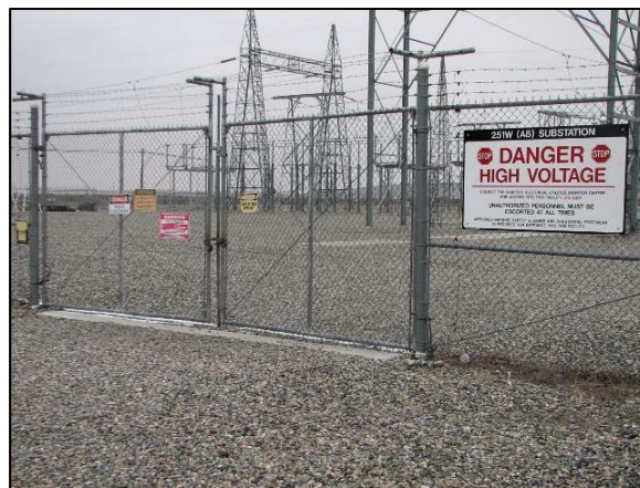
New Electrical Utilities signs posted at the main gates to each of the Substation Yards.
