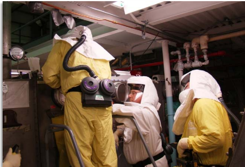
Activating HA-19B1 Gloveports in Room 235B
