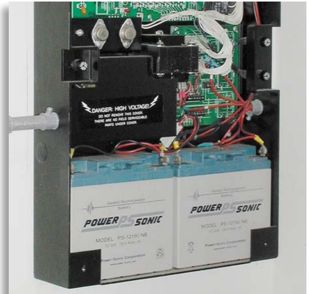
This fire alarm control panel employs batteries to provide its secondary power source.
