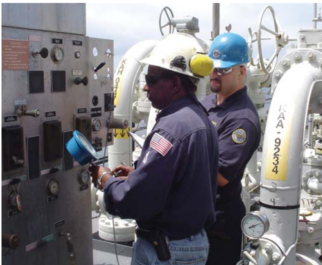
BOEMRE Inspector witnesses testing of safety device at instrumentation panel.
