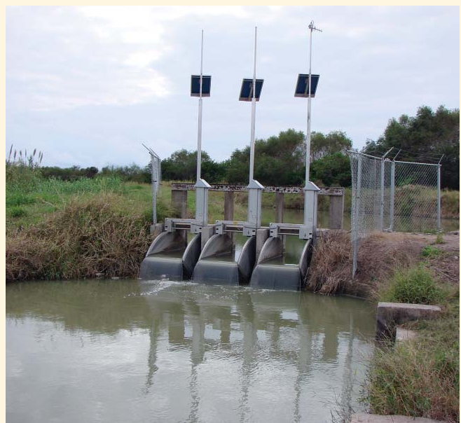
Replacement of manual gates with Rubicon standard programmable flume gate, Cameron County Irrigation District No. 2, TX, funded through the WaterSMART Grants program.
