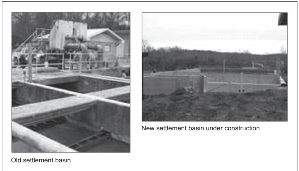
Figure 2: Old and New Settlement Basins at Montevallo, Alabama, Wastewater Treatment Plant
