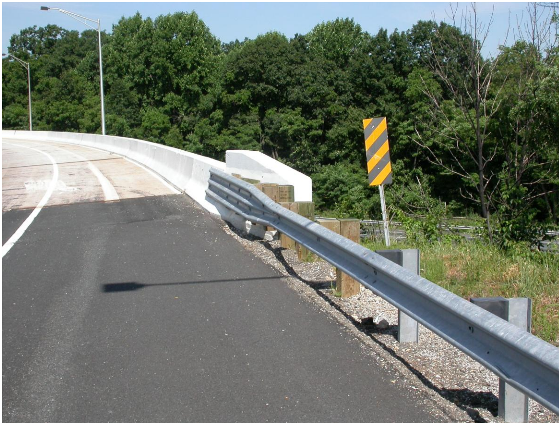
Figure 6. Postaccident modifications to the I-895 overpass barrier system.
