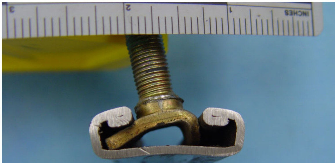
Figure 9. Damaged T-bolt in floor track.
