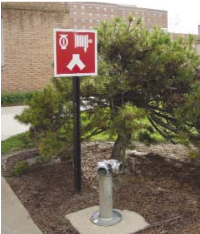
(Fig. 5.11) FDC sign with an NFPA 170 symbol for both sprinkler and standpipe systems.
