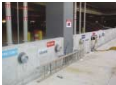
(Fig. 4.13) FDCs for separate manual dry standpipe systems in a large parking garage.
