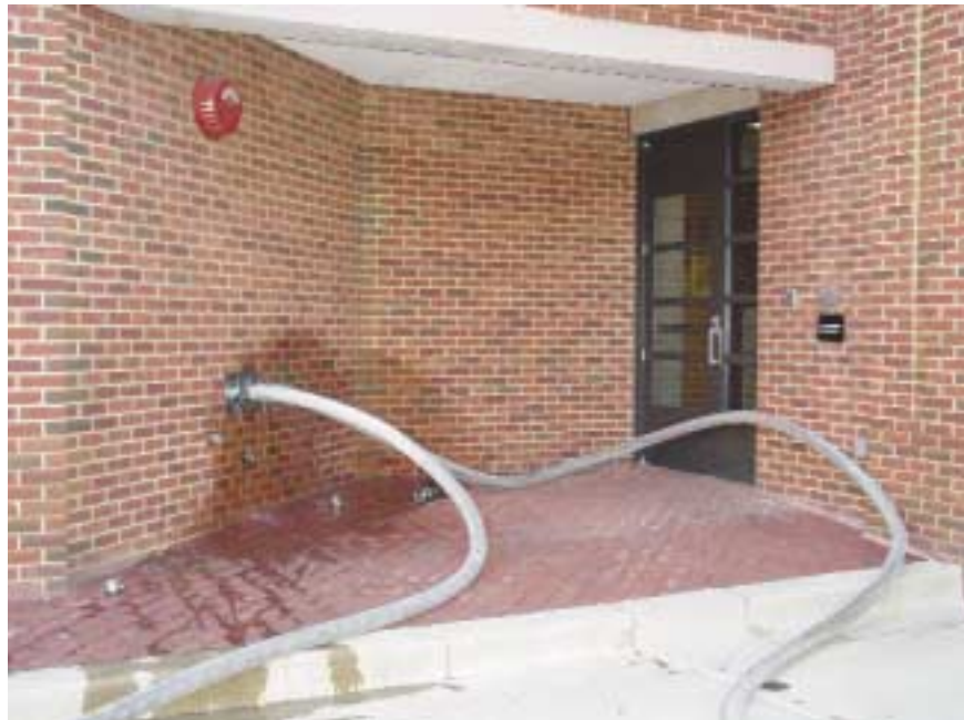
(Fig. 5.1) Charged hose lines connected to a wall-mounted FDC. The proximity of an FDC relative to building exits is discussed in the Location section at page 44.
