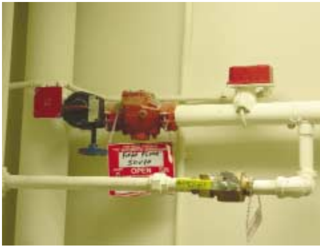
(Fig. 3.1) Sprinkler zone control station and zone indicator sign.
