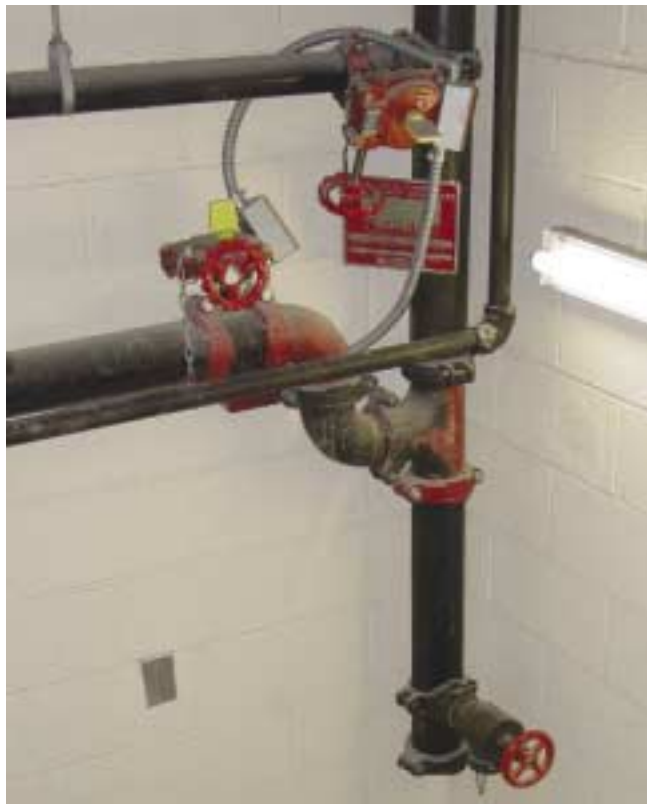
(Fig. 4.11) Isolation valve between the feed main (entering from the lower left) and the vertical riser (on the right). It is located within the stair enclosure for protection. The valve at the top of the photo is a sprinkler zone control valve.
