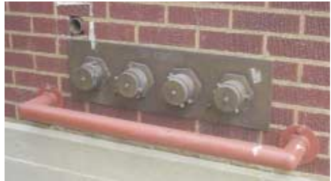
(Fig. 5.3) A 4-inlet FDC. It would probably be more efficient, and give the fire department more options, to have placed two, 2-inlet FDCs in different locations on this building.
