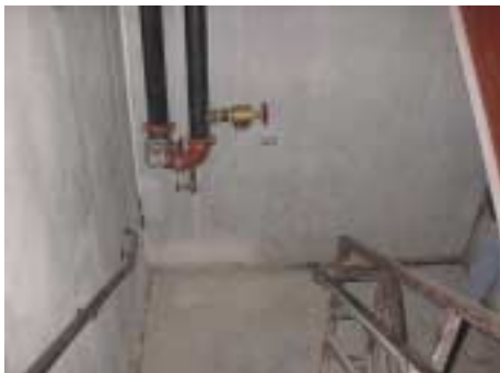
(Fig. 4.12) The feed for this standpipe was on a level above the fire department entry. The supply pipe was fed down (on the left) to the entry level, where the isolation valve was located. Then, the pipe was routed back upwards (on the right) to feed the standpipe riser.
