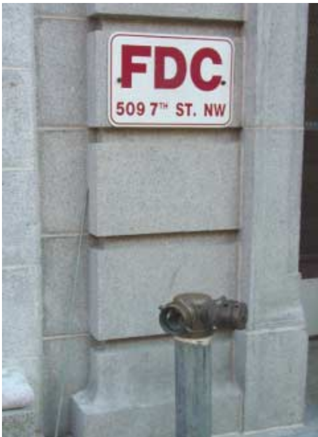
(Fig. 5.13) Address indicator sign to show which building this FDC feeds.
