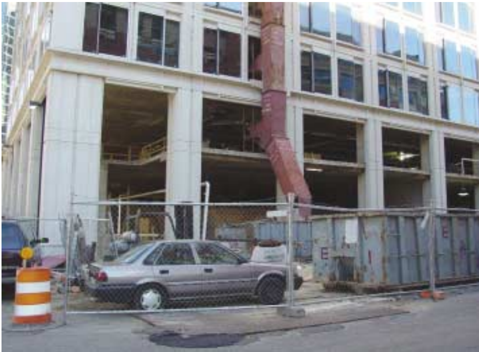
(Fig. 5.14) This is a building under construction as viewed from a piece of fire apparatus turning the corner onto the block. Can you see the FDC? It is not labeled, and it is blocked by a vehicle, a trash container, a fence, and construction materials. It is directly above the car's front bumper.
