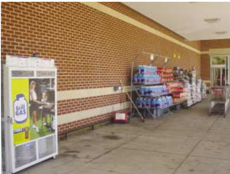
(Fig. 5.7) FDC in the cart area of a supermarket entryway. The FDC is located where merchandise or shopping carts could easily block it, or a fire in the adjacent propane storage area could restrict its use.
