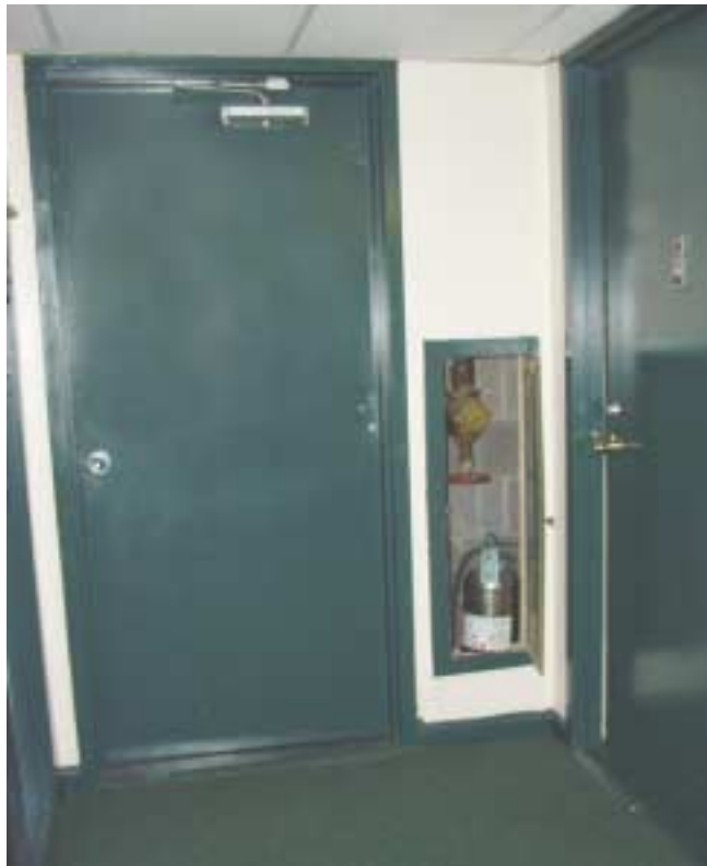
(Fig. 4.4) Hose connection on the corridor side of the stair door.
