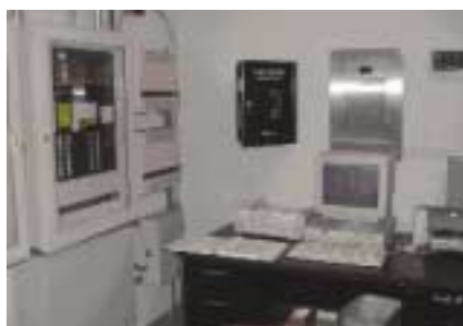
(Fig. 6.10) Fire command center with fire alarm and communications equipment, a work table, and adequate work space for the incident command staff.
