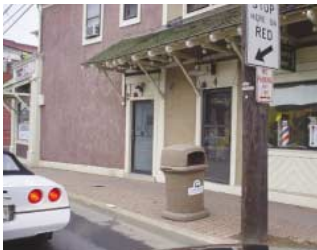
(Fig. 6.6) Strobes above each tenant entry door indicate the tenant where an alarm originates in this building, which has multiple tenants with different addresses fronting on two streets.
