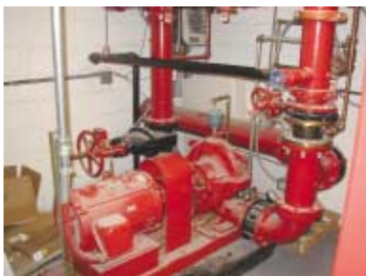
(Fig. 3.5) Fire pump.
