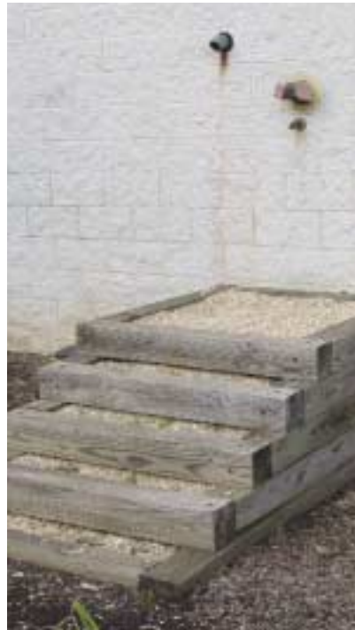
(Fig. 5.10) A platform built up to reach an FDC creates a hazardous condition. This should not be considered as equivalent to positioning the FDC at a proper height above grade level.
