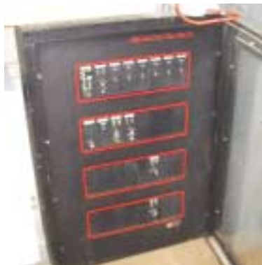
(Fig. 6.1b) Control panel.
