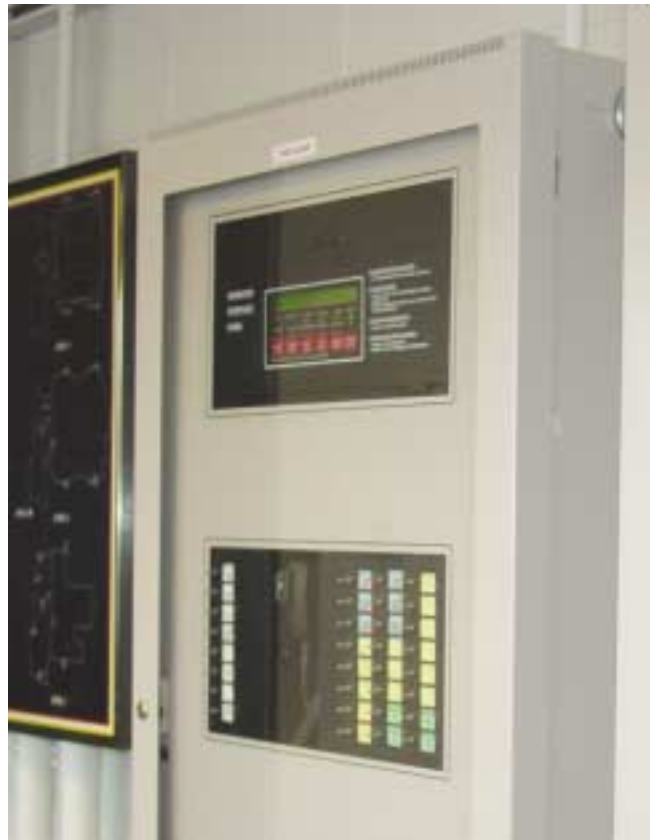
(Fig. 6.7) The grey panel is a voice alarm panel. The lower window shows the microphone and the manual select switches for the different evacuation zones.
