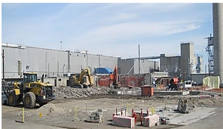
The site of the former 2736-ZB Vault Complex at the Plutonium Finishing Plant
