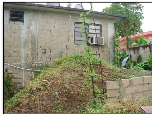
Assistance in the amount of $3,951 was approved for the construction of a new bedroom in the back of the existing dwelling unit. However, the entrance to the new bedroom would be through an existing bedroom.
