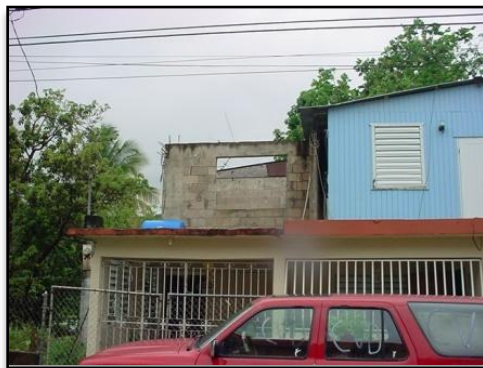
Assistance in the amount of $3,215 was approved for the construction of a new bedroom on the second floor of the existing dwelling unit. However, the scope of the rehabilitation work did not include the construction of a protecting wall or fence to avoid falls from the second floor.
