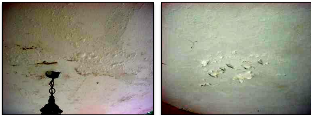
The above pictures show deficient rehabilitation work paid for with Block Grant funds. Water leaks still existed in the dwelling units when we conducted our inspections.
