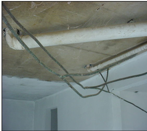
Water lines were hanging from the living room ceiling.
