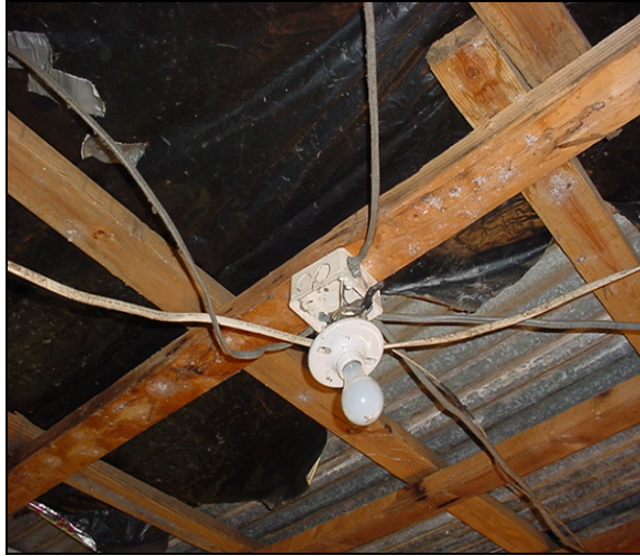
An improper electrical connection and missing ceiling panels created a safety hazard.
