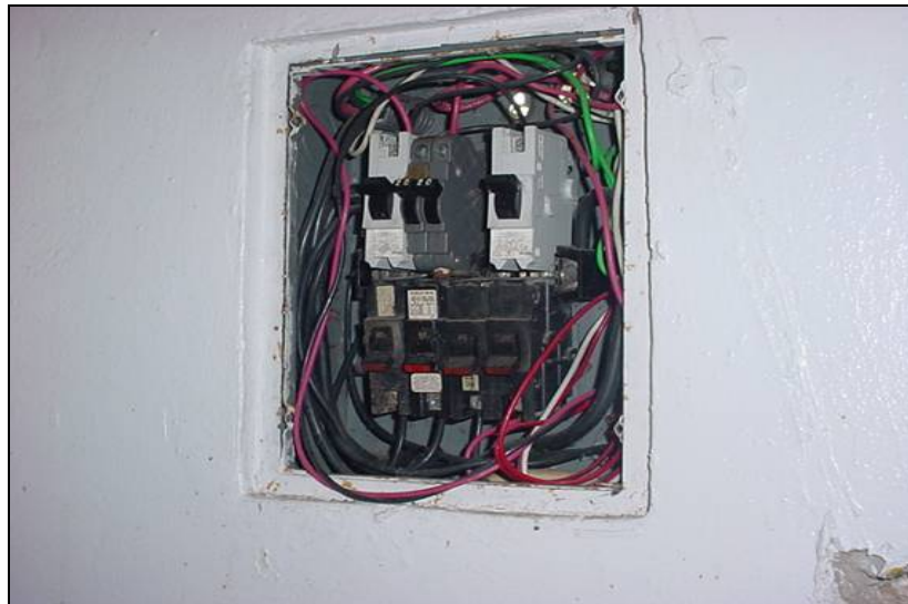
Breaker panel with no internal fixed cover and with exposed electrical contacts, creating an electrical shock hazard.
