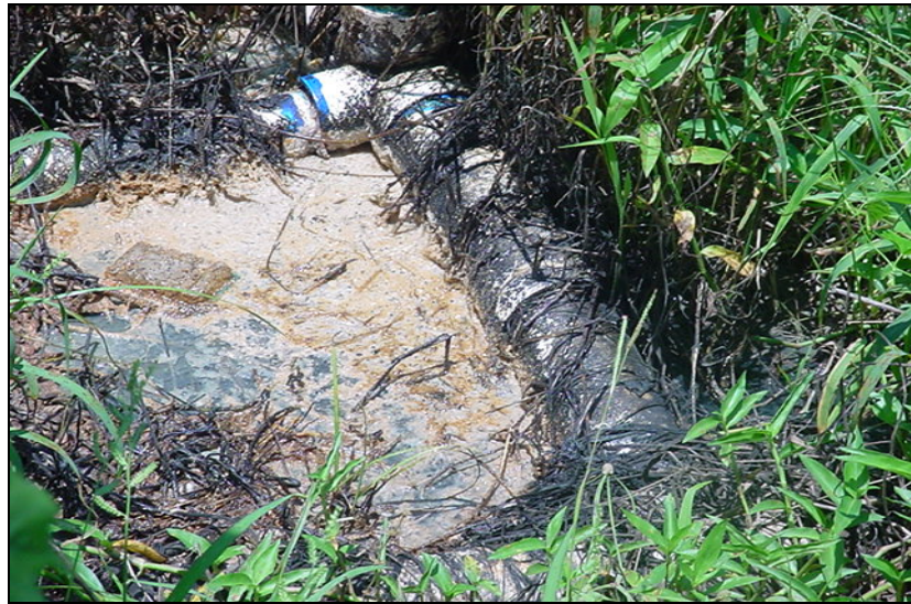
Raw sewage spill from defective septic tank in the back of the dwelling unit.
