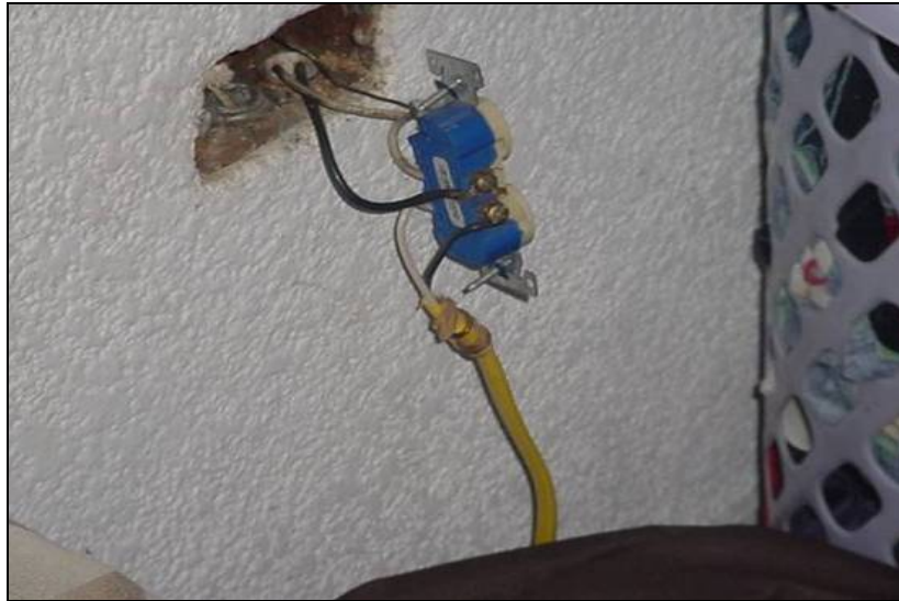
Electrical connection with exposed wires, creating an electrical shock hazard.
