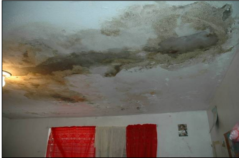
Peeling paint and serious water leak on living room ceiling.
