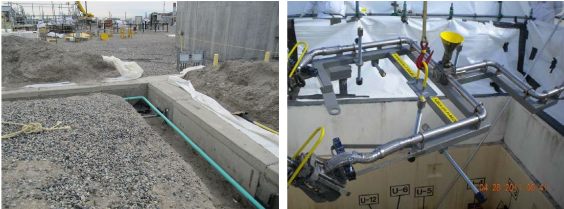
Figure 3-2. 241-AZ Condensate Line
