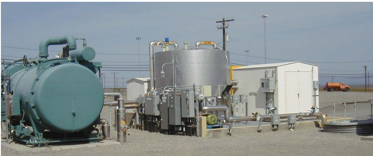
Figure 4-1. Project W-211 Installed Diluent and Flush System, West of AN Farm
