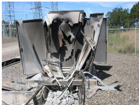
Figure A-1.1 Collateral Damage from Attempted Metals Theft
