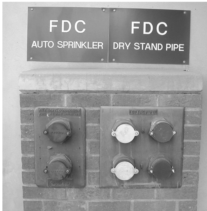
Figure 3-6 Preincident Planning Fire Department Connections Eliminate Confusion
