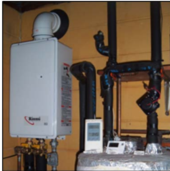
Figure 48. Tankless water heater elevated above 80-gal storage tank (lower right)
