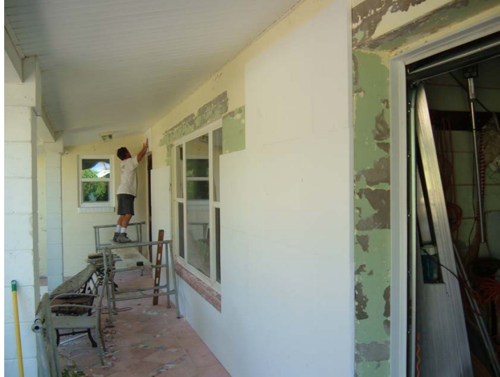
Figure 65. Exterior EIFS wall insulation retrofit in progress. Insulation consists of 1 in. of expanded polystyrene on the exterior covered by fiberglass mesh and vinyl texture stucco.
