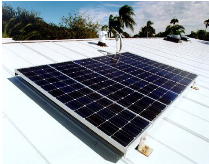
Figure 66. 450 W of solar modules powers pool pump directly. Solatube on white metal roof can be seen in the background. Array shown before installation of larger 4.9-kW PV system.
