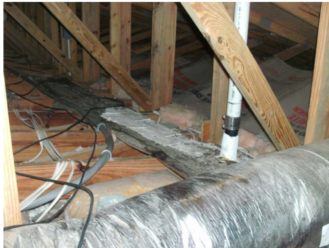
Figure 68. Attic ducts, while sealed, are only insulated to R-6 and a major source of heating system heat loss in winter and cooling season heat gain in summer. Using the mini-split allows the duct system to be largely abandoned in place without these losses for space conditioning.
