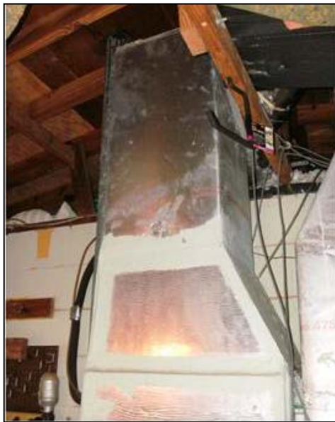
Figure 7. A/C evaporator and plenum showing segments sealed with mastic
