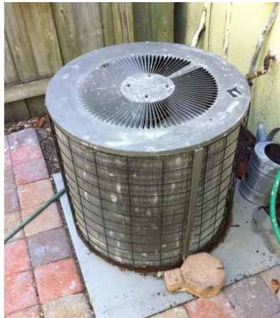
Figure 5. Outdoor unit for SEER 10, 2-ton A/C installed in 1995 and still in use
