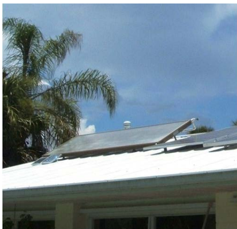
Figure 47. 4 ft × 8 ft solar collector. System is PV pumped by two 5-W PV modules mounted in parallel.
