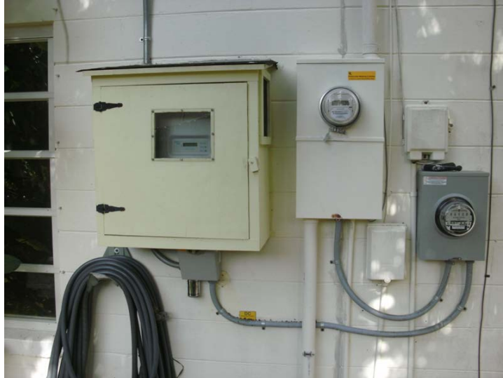
Figure 74. SMA 5000-W inverter is located on the east side of the home with the utility bidirectional meter. A ventilated enclosure was built to protect the inverter from sun and rain.
