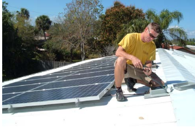
Figure ES-1. 4.9-kW rooftop PV system is connected in February 2009. The white metal roof was part of house improvements in the 1998 remodel.
