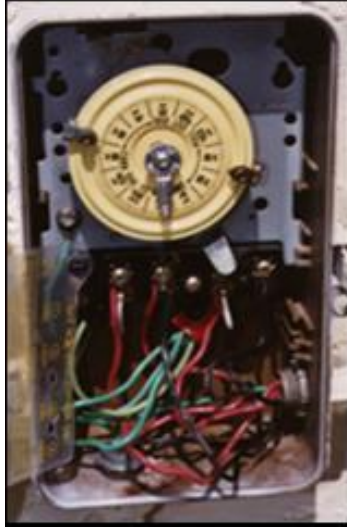
Figure 4. Pool pump timer. Immediately after taking over the house, this was set from 8 h/day to only 3–4 h/day, saving an estimated 2000 kWh annually.
