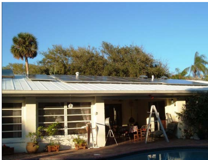
Figure 75. South roof of the home showing 4.92-kW PV system, 450-W PV pumping array, and solar water heating system (far left).
