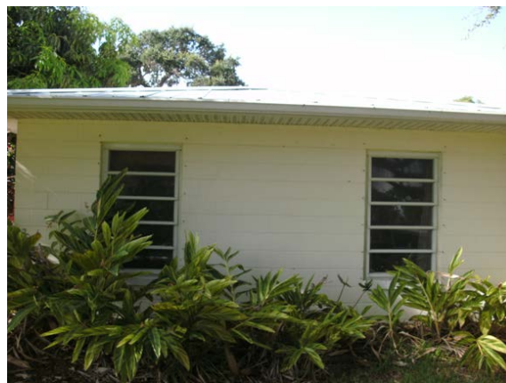
Figure 62. Poorly fitting single-glazed awning windows with aluminum frames before retrofit
