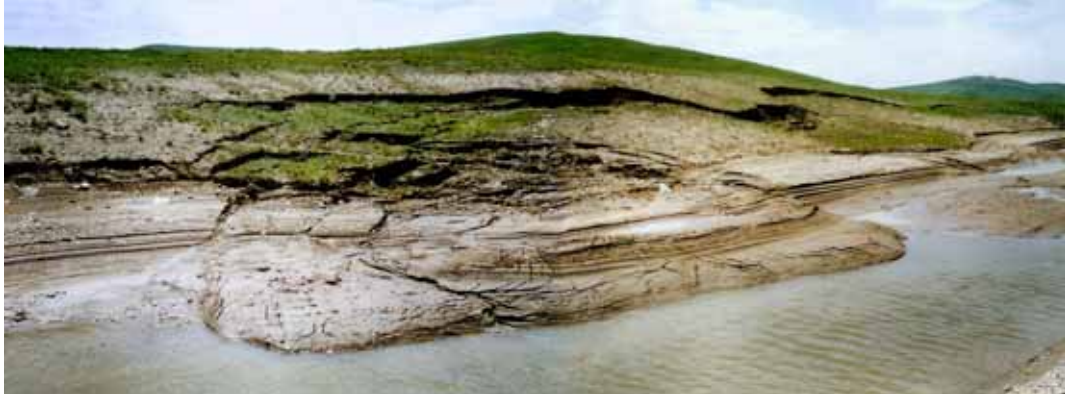
Figure 5.4: One of 16 documented slides on the St. Mary Canal.
