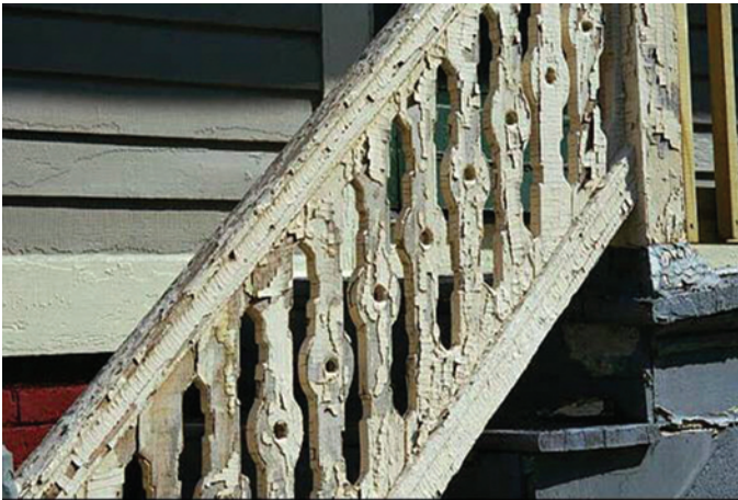
Outdoor stairs to a house featuring a banister with badly peeling paint.
