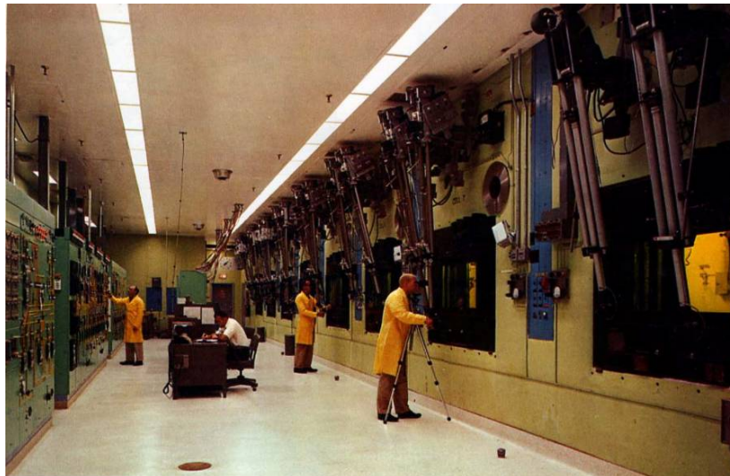
Fig. 52. The operating gallery of the Transuranium Processing Facility.
