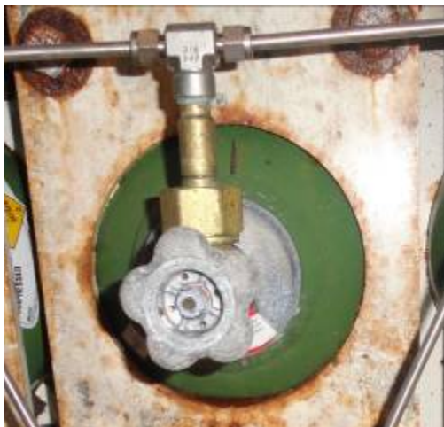
Figure 1 – View of Installed Fitting
