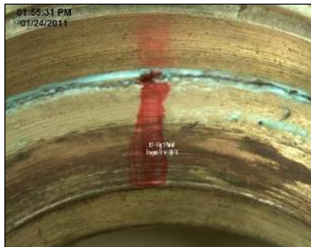
Figure 2 – magnified view inside brass fitting showing cracking (this fitting was still intact and held compressed gas)
