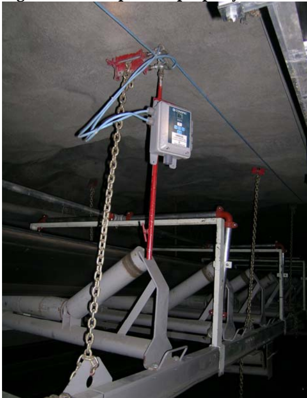
Figure 1 - Example of a properly installed CO sensor.
