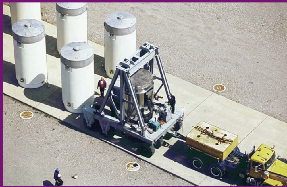
Dry casks for spent fuel are transported and placed on a concrete pad at a nuclear plant site.
