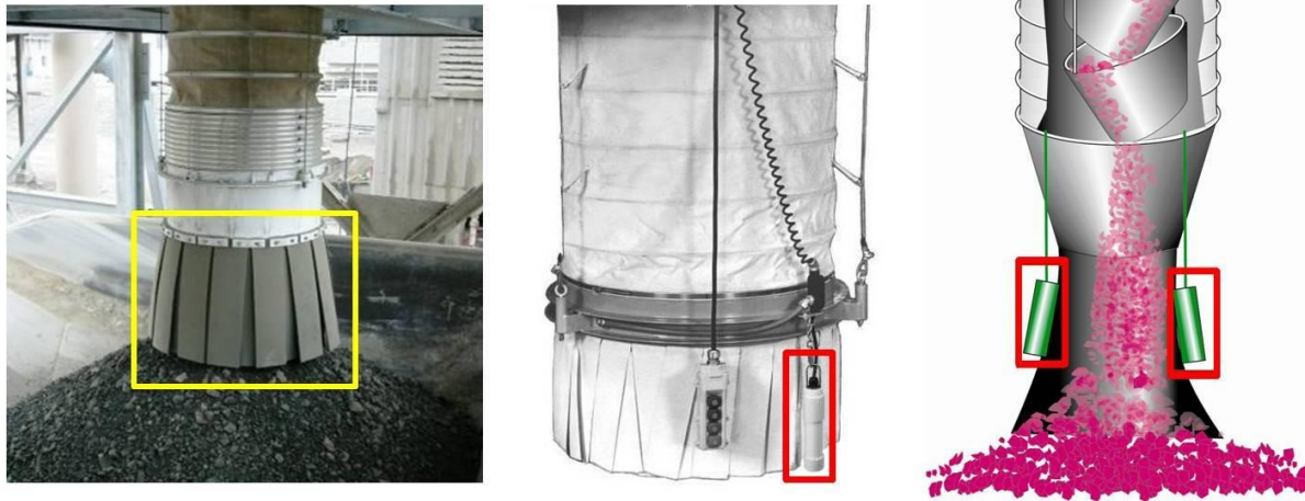
Figure 7.4. Skirt (in yellow box) and tilt sensors (in red boxes) installed on the discharge end of loading spouts to help reduce dust emissions.
