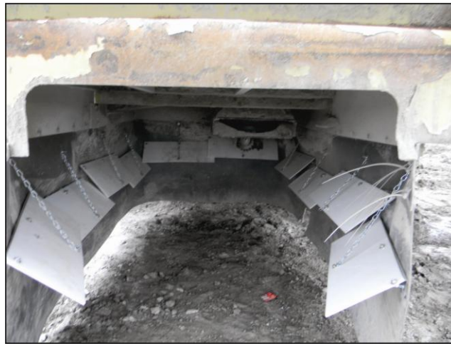
Figure 3.12. Air-blocking shelf with modifications incorporated into installation. This shelf was installed in short sections in an attempt to prevent potential damage that could occur during tramming with the drill mast up. Note that each of the sections overlap, eliminating any gaps in the shelf perimeter.
