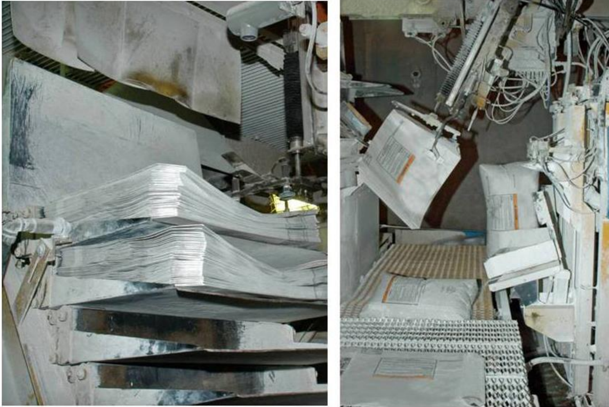
Figure 6.13. Bag storage shelves shown on left; a robotic arm with suction cups to place empty bags on fill nozzle shown on right.
