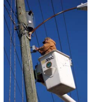
Figure 4: Sensor Installation in Newport News
