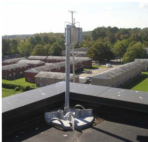
Figure 14: SECURES ® Sensor Installed On 11th story roof top with ballast mount
