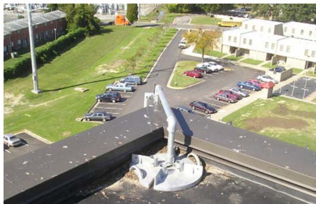
Figure 13: SECURES ® Sensor Installed On 11 th story roof – with ballast mount at roof line
