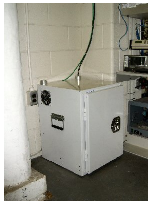
Figure 7: NNPd SECURES Receiver Station
