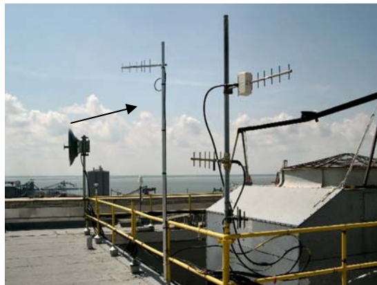
Figure 6: NNPd SECURES Receiver Antenna
