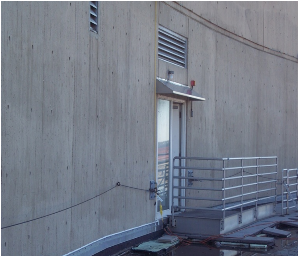
Figure 1 – Unsecured door on Weaver Building rooftop after business hours.
