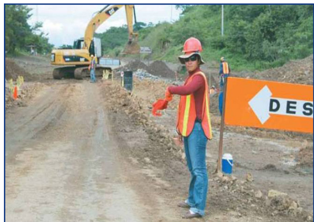
MCC and its partners support expanding women's employment opportunities in its infrastructure projects.
