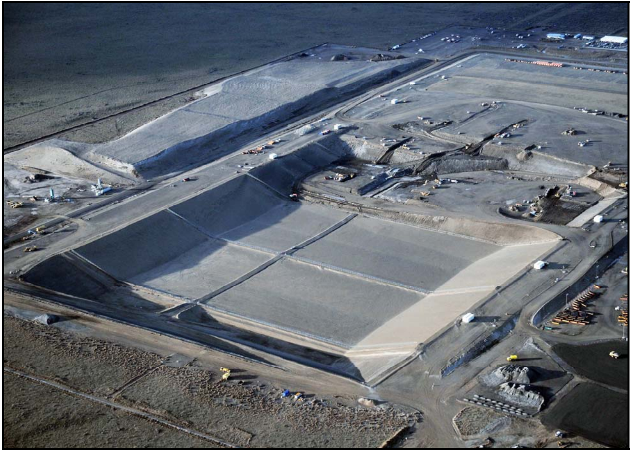
An aerial photo from the northeast corner of the Environmental Restoration Disposal Facility shows super cells 9 and 10 after construction was completed. (Photo 1)
