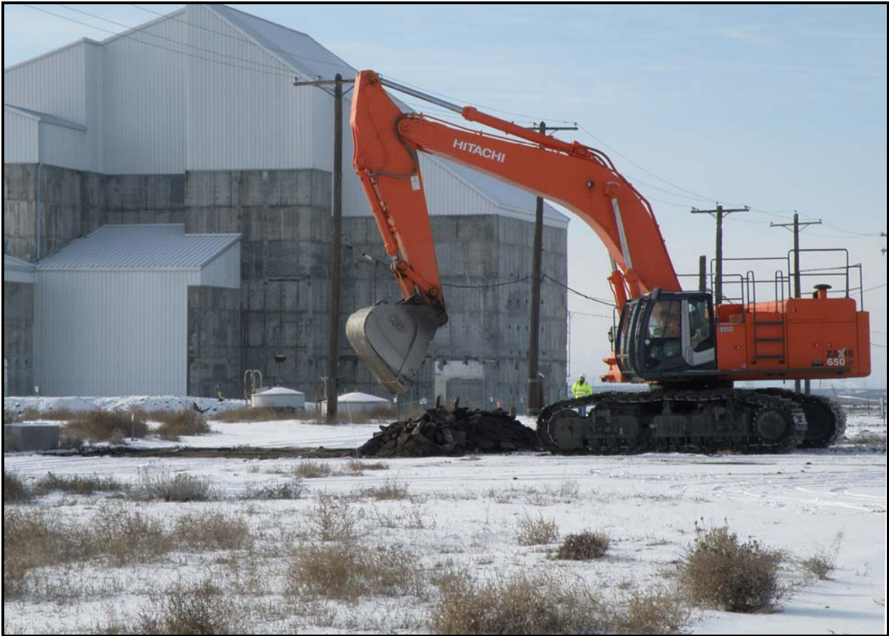
Washington Closure Hanford subcontractor Ojeda Business Ventures began removing overburden at 100-F-26:7, a site that contains sodium dichromate and sodium silicate pipelines. (Photo 7)
