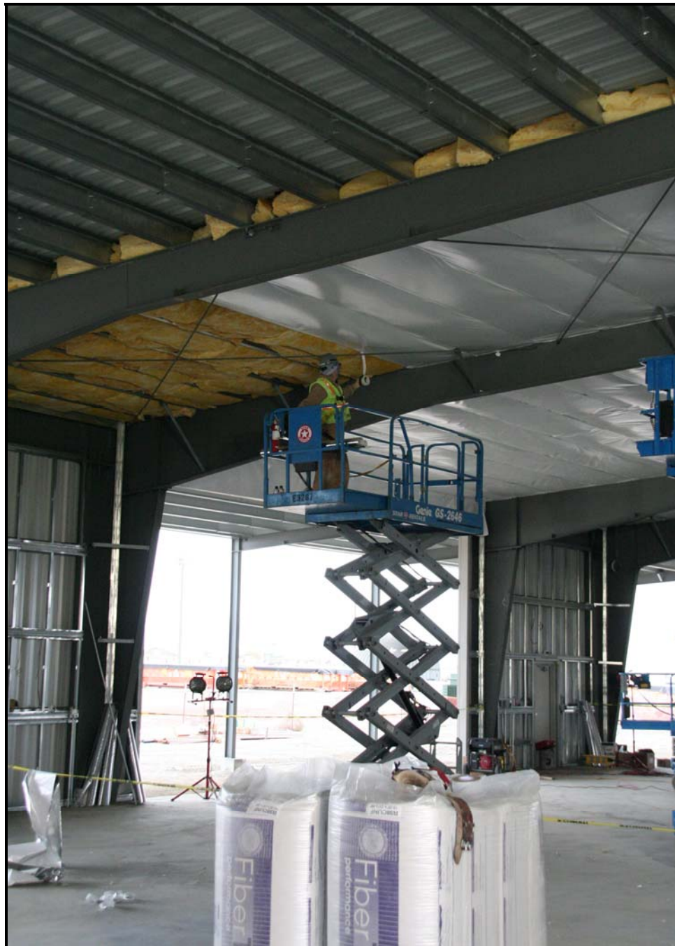
Washington Closure Hanford subcontractor ELRFowler installs insulation in the container maintenance facility. (Photo 2)
