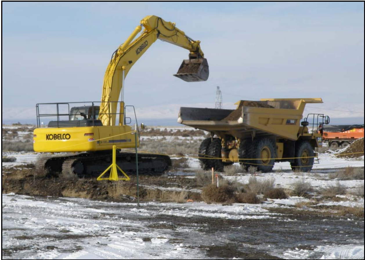
Ojeda Business Ventures performs excavation and stockpiling at 100-F:49. The site consists of an old maintenance garage lube pit foundation, pipelines, and drywells. (Photo 8)
