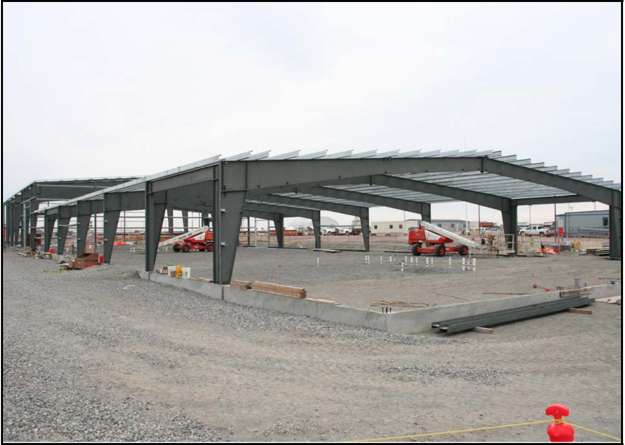
ELRFowler completed erection of the steel skeleton of the equipment maintenance facility/operations center. (Photo 3)
