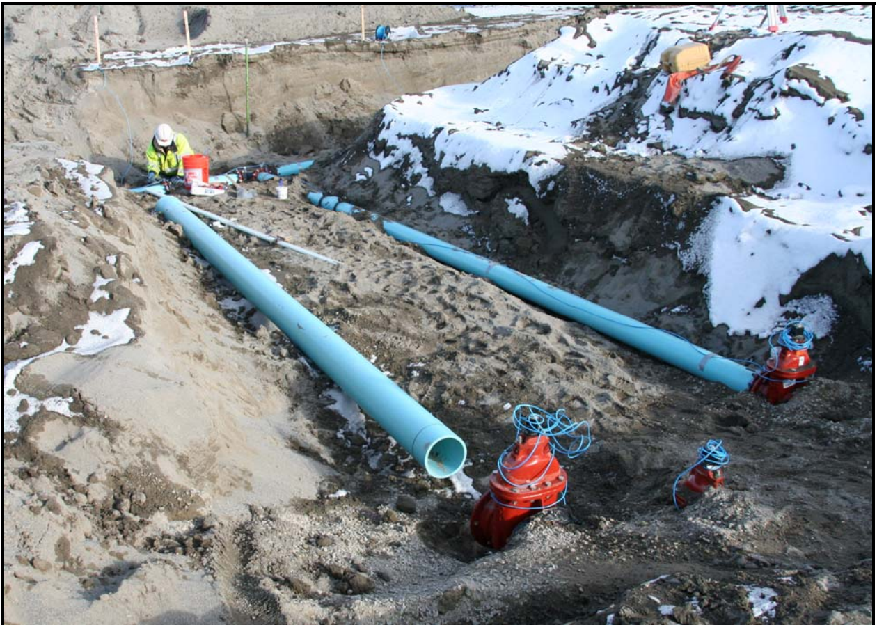
Washington Closure Hanford subcontractor White Shield/Apollo installs piping to water tanks at the 618-10 Burial Ground. The water will be used for fire suppression and dust control. (Photo 4)
