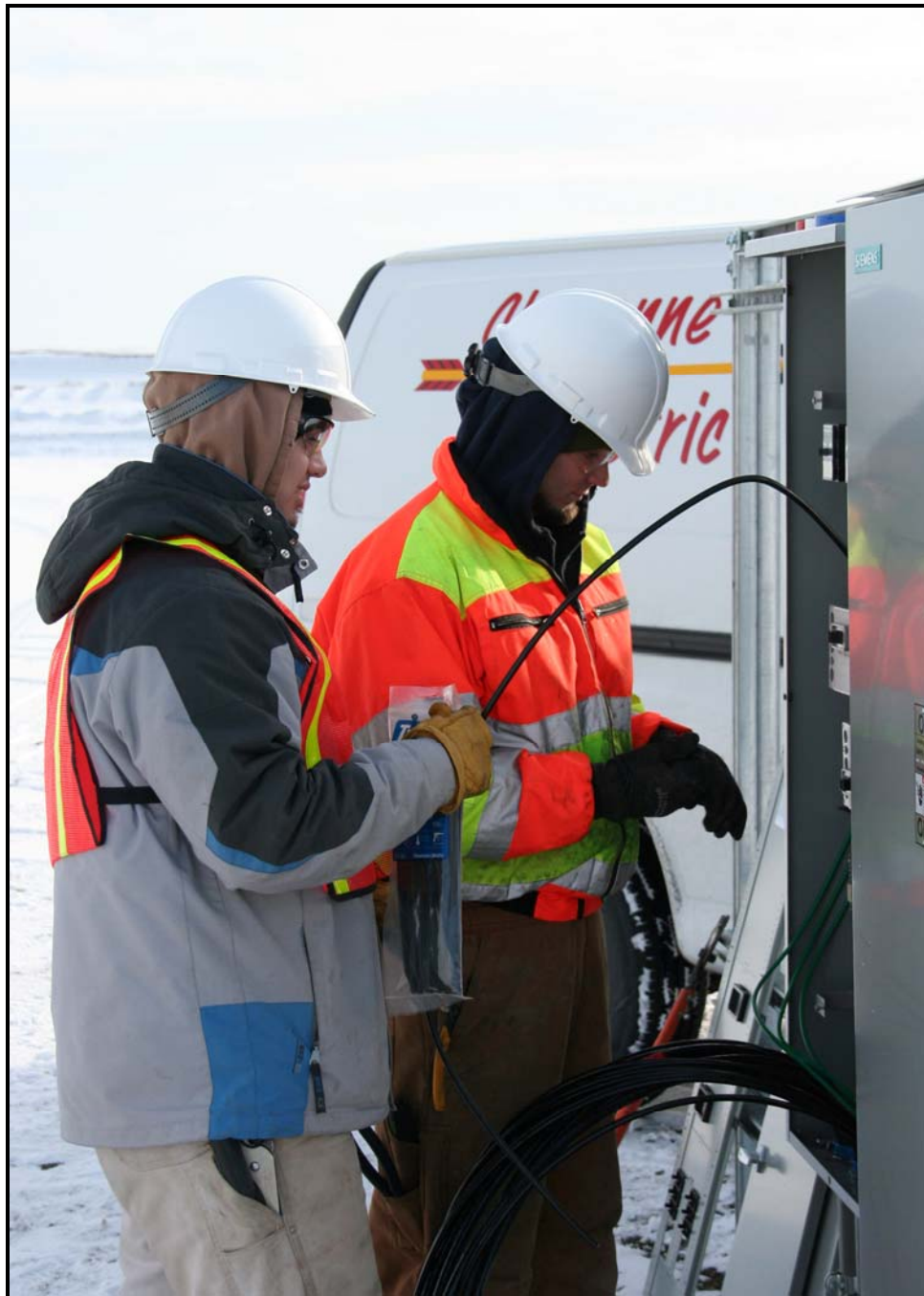
Workers install electrical at the container staging area of the 618-10 Burial Ground. (Photo 5)
