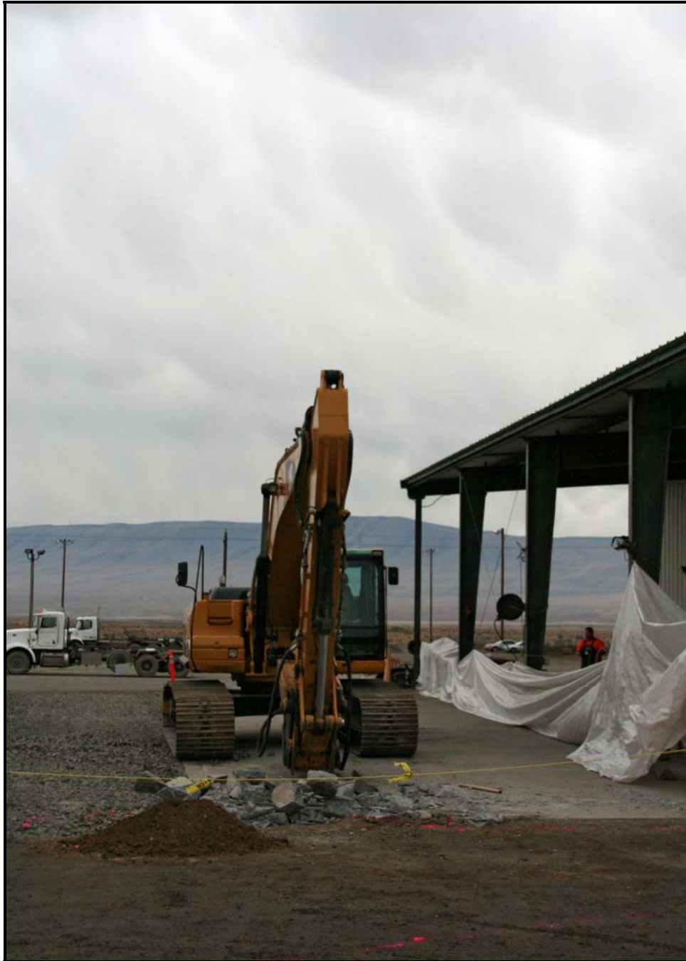
Fowler General Construction begins to break up the concrete pad at the existing truck maintenance facility. The current facility is undergoing expansion. (Photo 4)
