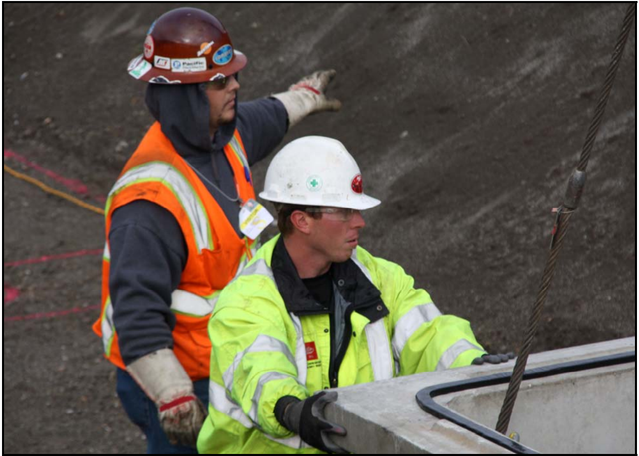
White Shield/Apollo workers position a septic tank at the 618-10 Burial Ground. (Photo 7)
