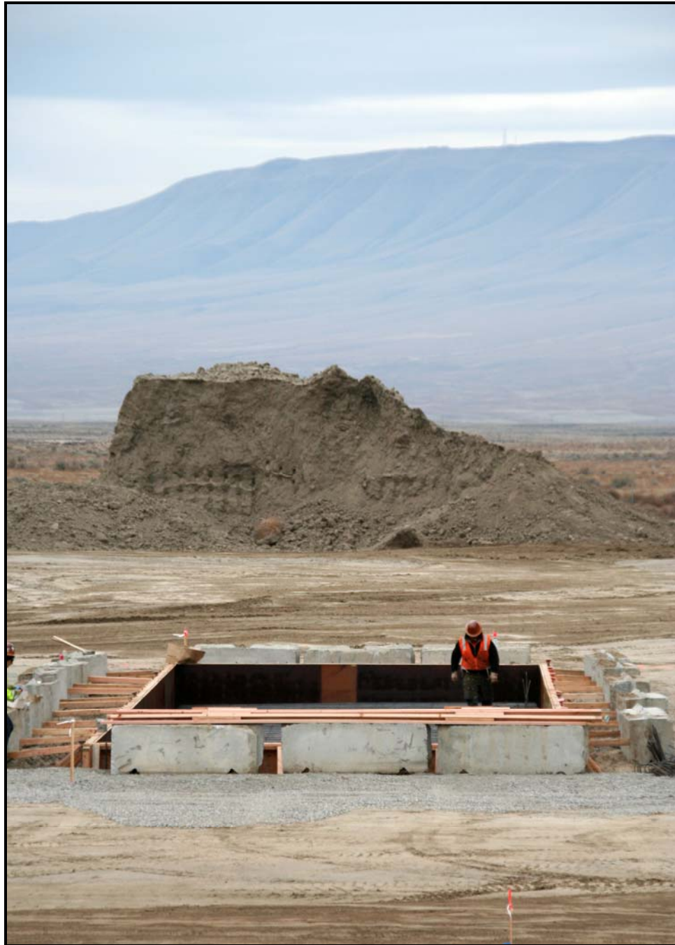
Washington Closure Hanford subcontractor DelHur Industries workers prepare to pour the foundation for the new batch plant at the Environmental Restoration Disposal Facility. (Photo 5)
