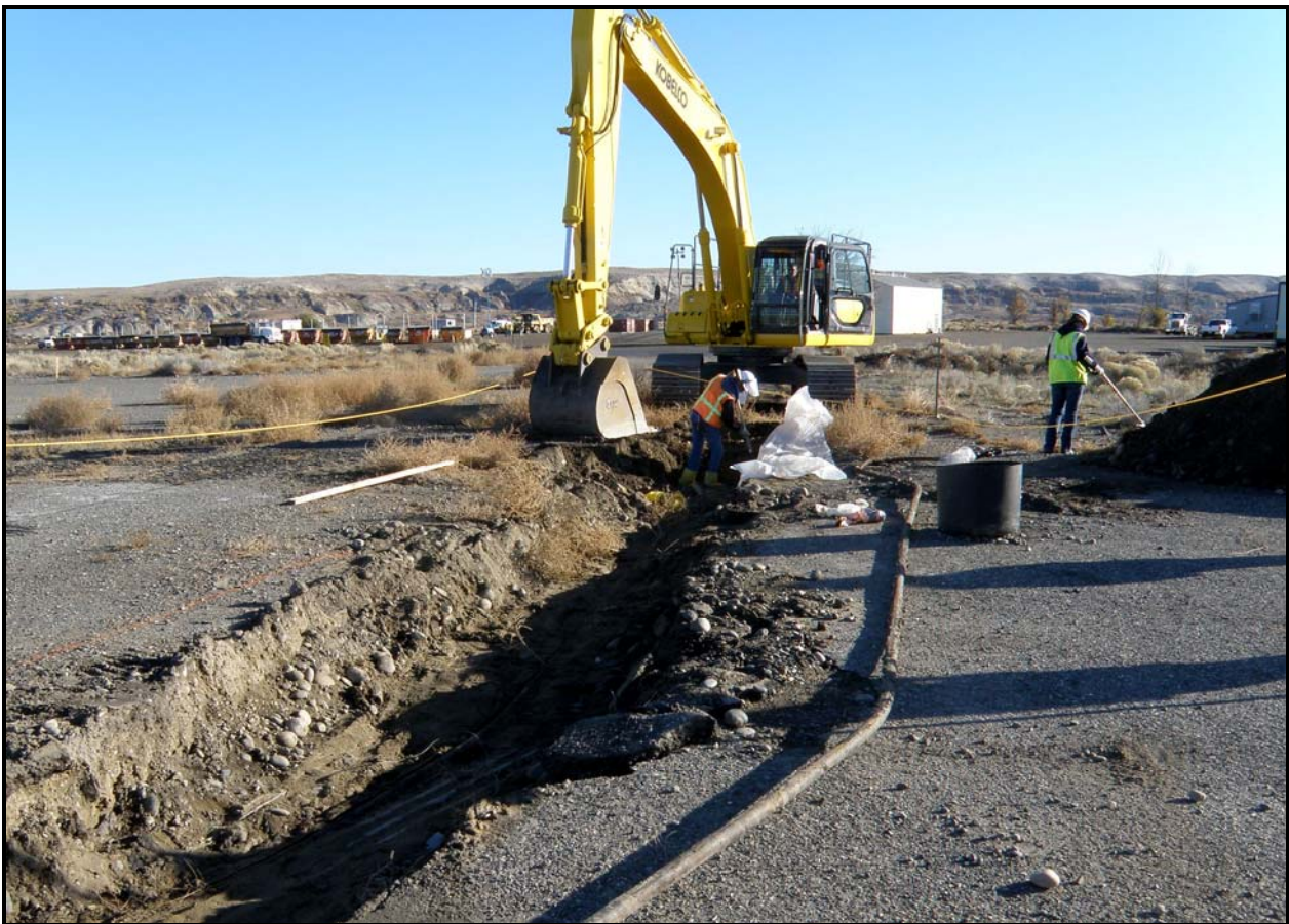
Washington Closure Hanford subcontractor Ojeda Business Ventures completed excavation and loadout activities at 100-F-44:8, a site that contained old fuel pipelines. (Photo 9)
