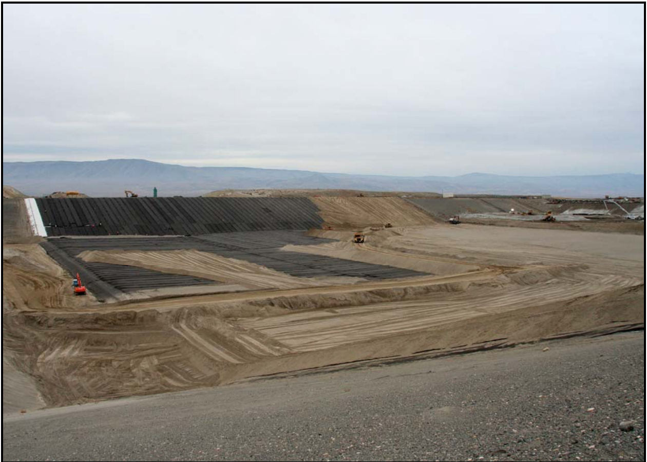
A view from the northeast corner of super cell 10 shows construction progress at the Environmental Restoration Disposal Facility. (Photo 1)
