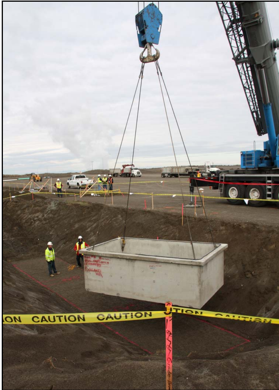
Washington Closure Hanford subcontractor White Shield/Apollo lowers the first of three septic tanks into place at the 618-10 Burial Ground. (Photo 6)
