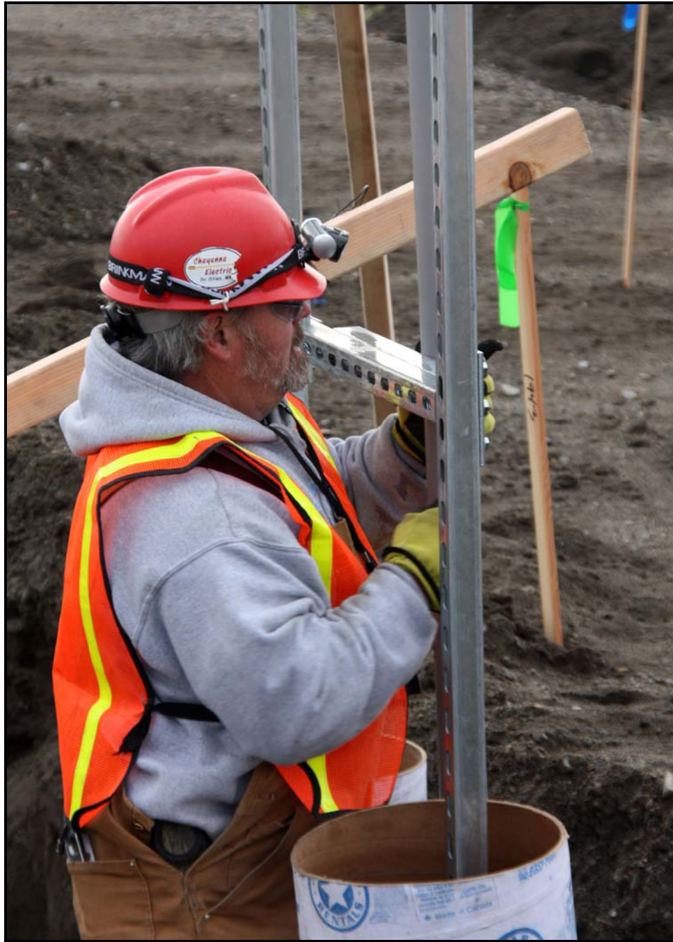
Work continues to install conduit for the electrical at the 618-10 Burial Ground. (Photo 8)
